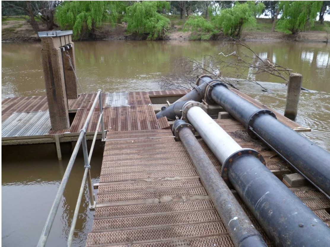
Plate 3 – Raw water intake pipes
