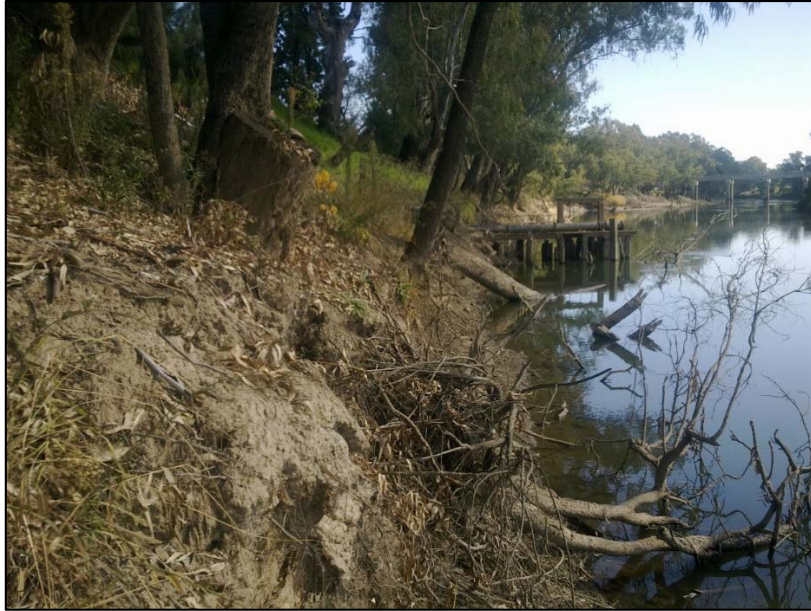
Photo 8: View of eroded south bank, looking west towards existing river intake
