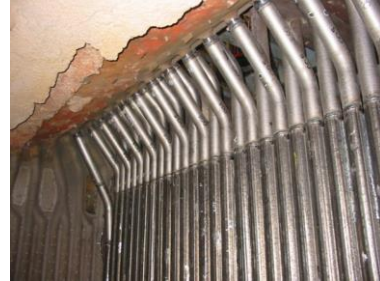
Fig. 5.5 f – Connecting piping between the boiler drum and membrane wall (KRB)
