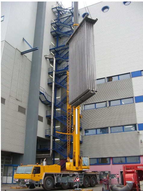
Fig. 5.5 b – Hoisting of a replacement superheater tube bundle with a mobile crane to the top of the boiler building for installation during annual overhaul (KRB)
