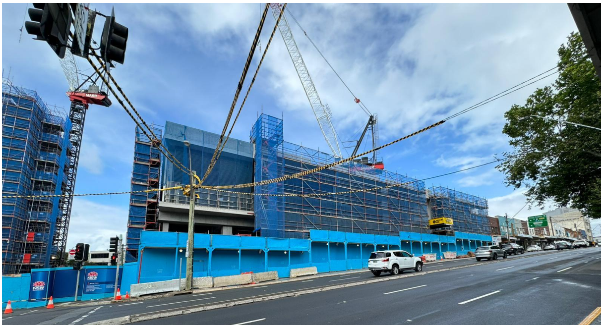
Figure 17: View looking north-east towards the subject site, at the intersection of Pacific Highway and Hume Street. The construction of the Crows Nest Metro Station podium was underway during the site inspection in October 2023.
