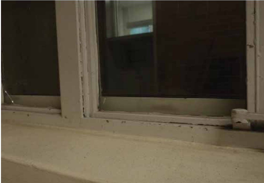
Photo 11 - Internal Window Paint Blackburn Building
