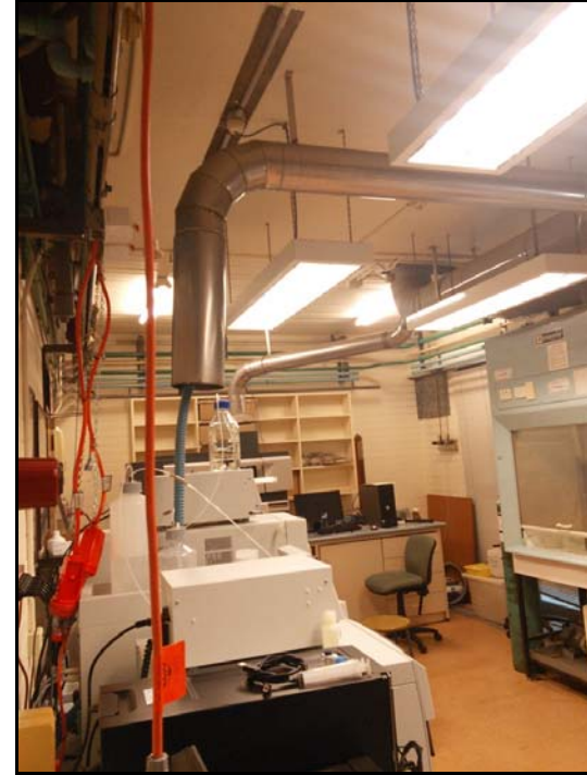
Figure 4 – Building J01 Embedded Equipment
