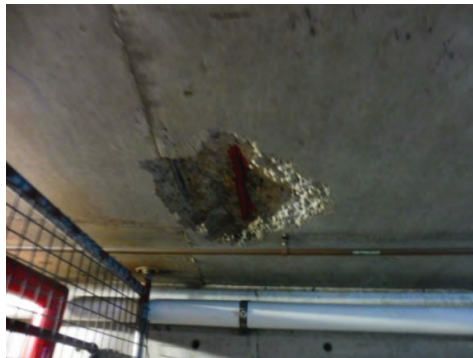
Spalling concrete to soffit B3
