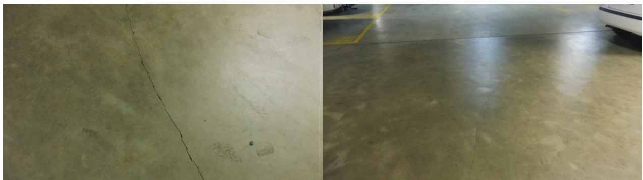
Local cracking to B2 floor
