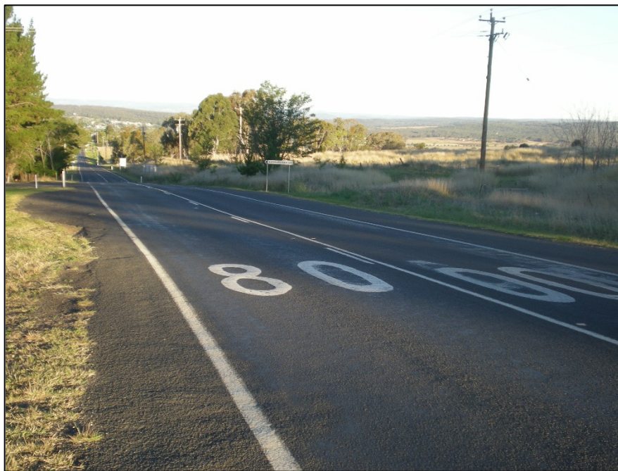
■ Photo 9 Example of non-conforming sealed shoulder width on Gwydir Highway approximately 1km east of Bindaree Beef site (towards Inverell town centre)
