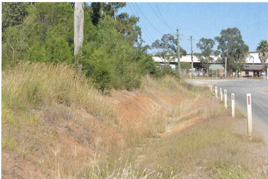
Figure 3.7 View E. Excavations have cut the natural landforms for road construction. (Source: GML 2014)
