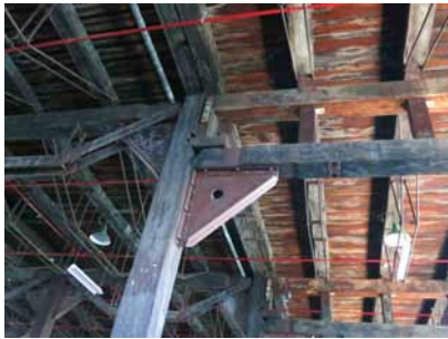
Figure 2.4.13: Pier 2/3 Ground floor, evidence of first floor deck raised along western edge
