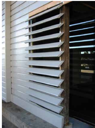
Figure 7.4.3: Weatherboards used as louvres in a fixed position. This option is not proposed at Pier 2/3.
