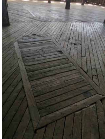
Figure 2.4.18: Pier 2.3 Ground floor, evidence of hatch blocked up.
