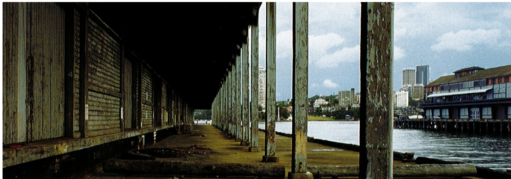
Figure 3.1.3: Decaying state of Pier 6/7, while Wharf 4/5 (seen right) flourished (Source: Field, N and Walker, C, 'Walsh Bay: Harbourside Renewal')
