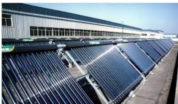
Figure 1 Solar Hot Water Roof Mounted Collectors
