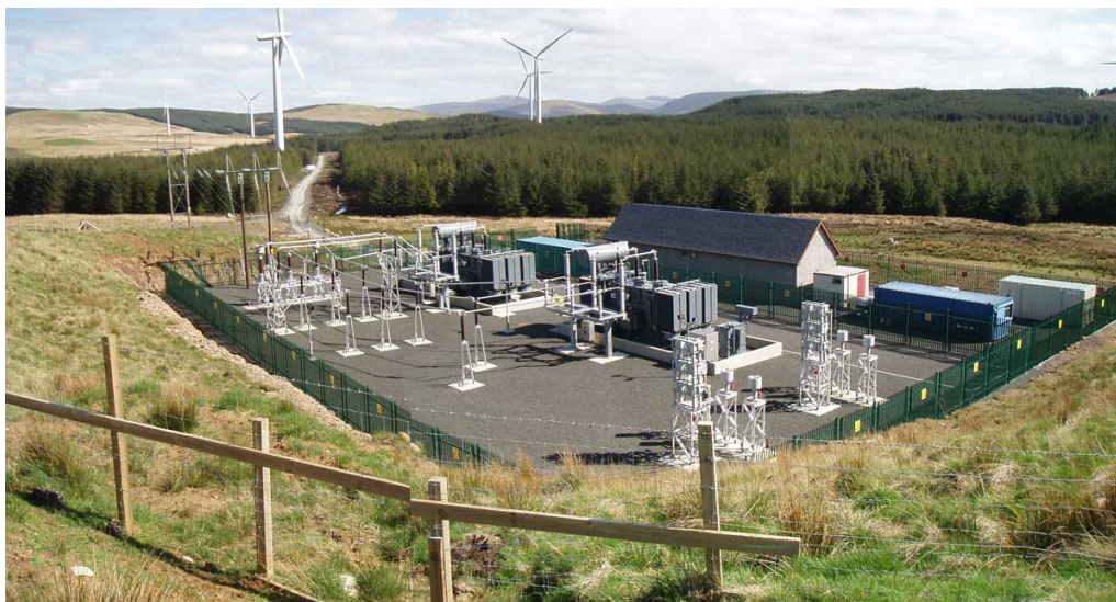
Photograph 3-2 Typical Wind Farm Sub-station (Source: DP Energy 2010)
