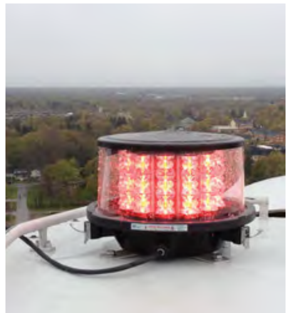
Typical WTG obstacle lighting
