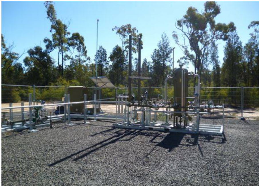
Plate 3-1 Typical wellhead separator
