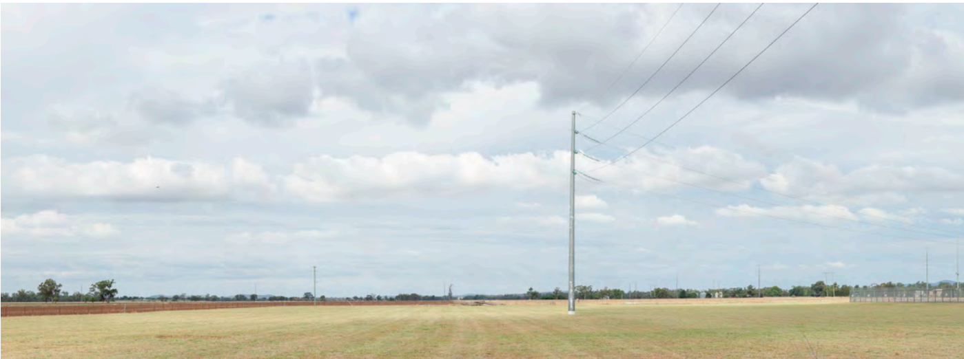
Image 06 132kV Overhead Transmission Line
