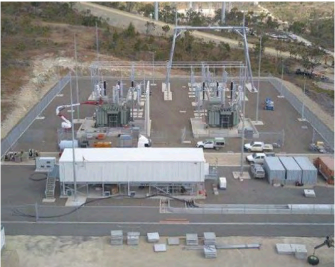
Image 05 Typical Substation (Source: ERM)
