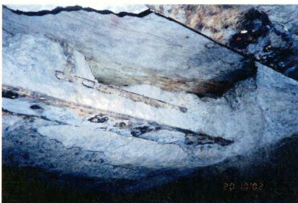
15. DC30P1-CP01 (Ch 104.0) Exposed steel beams in roof
