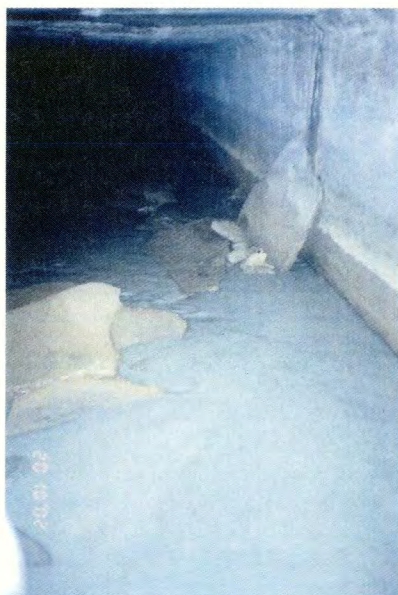
7. DC30A2-CP11 to CP14 (Ch 91.0) Debris in channel floor
