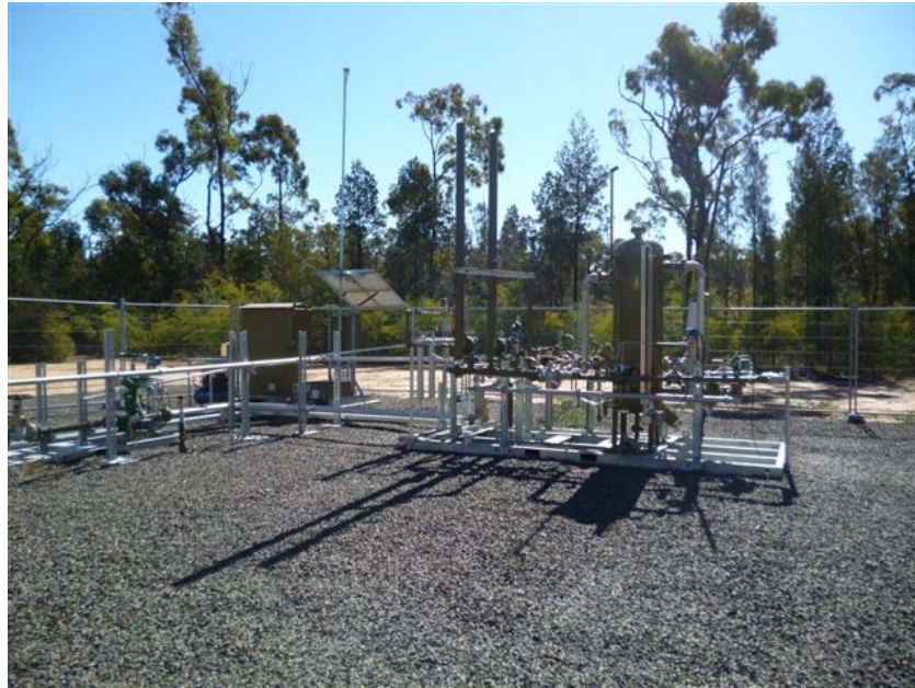
Plate 4-1 Typical wellhead separator and metering skid
