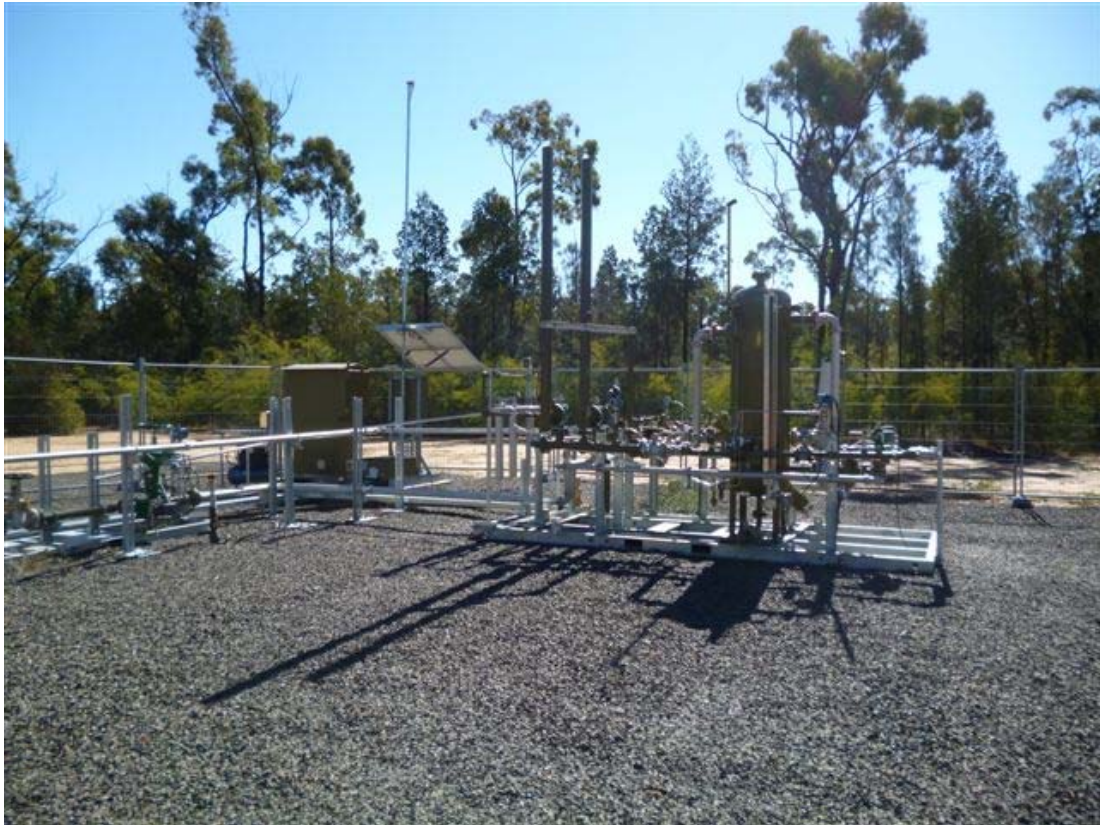
Plate 3-1 Typical wellhead separator
