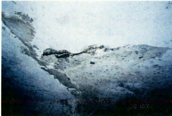
9. DC30P1-CP07 to CP08 (Ch 118.0) Spalling concrete & exposed reo
