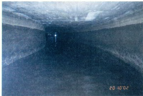
14. DC30P1-CP04 (Ch 0.0) Heavy silt just below waterline
