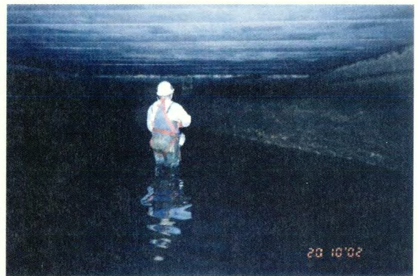
12. DC30P1-CP05 (Ch 332.0) Transition & weir across DC30P1
