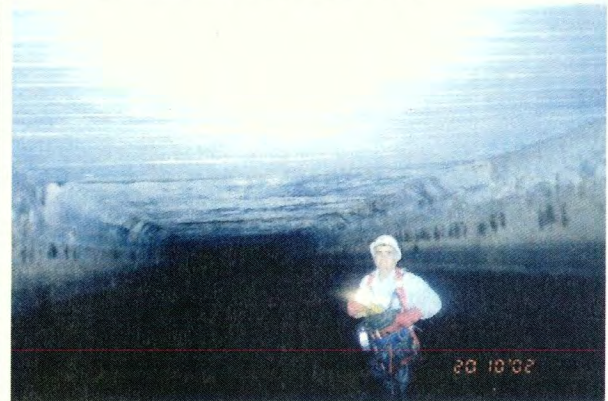
10. DC30P1-CP07 to CP08 (Ch 132.0) Aluminium sheeting in roof
