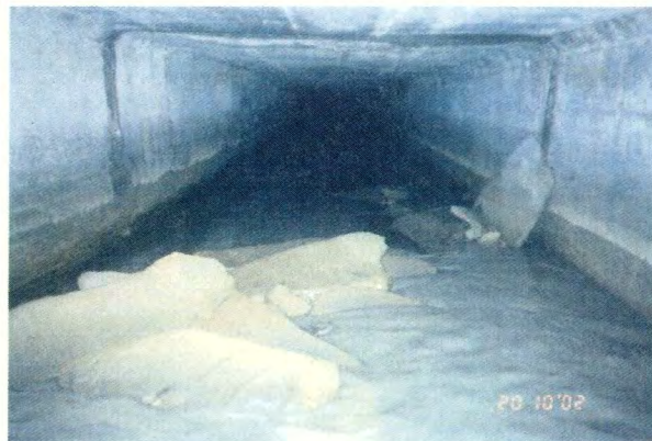
6. DC30A2-CP11 to CP14 (Ch 91.0) Debris in channel floor
