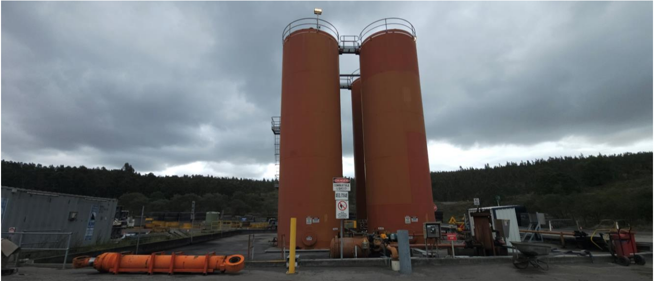
Image 5: Bunded above-ground tanks at the Workshop
