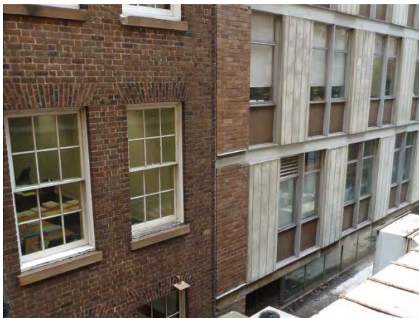
Figure 3.18 View of the connection between the Wynyard Lane facade of Beneficial House (on the left) and 301 George Street (on the right). (Source: GML 2014)
