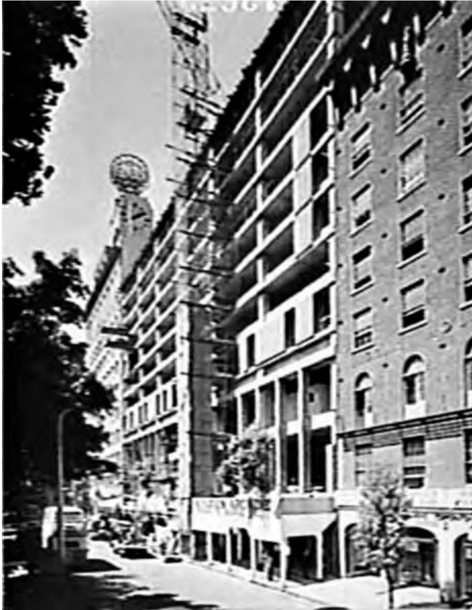
Figure 2.42 1963 Menzies under construction. Note what appears to be the Shell sign on top of the Shell House Clock. (Source: SLNSW d7_13672r)
