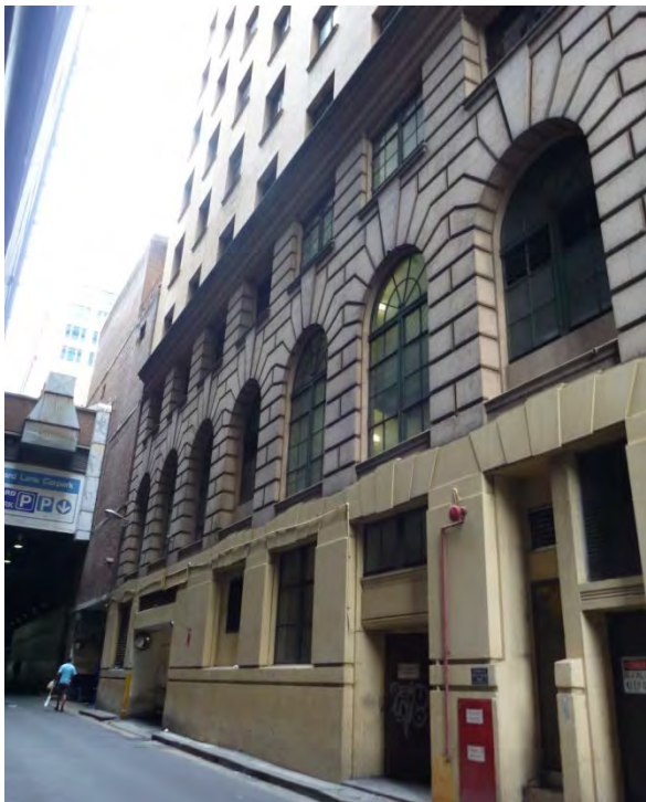
Figure 3.8 Wynyard Lane facade of the former Shell House, showing rendered masonry, and original steel-framed windows (Source: GML 2014)
