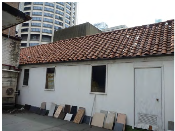
Figure 3.19 The store room on the roof of Beneficial House, contained beneath the parapet with tiled, gable roof to the George Street facade. (Source: GML 2014)
