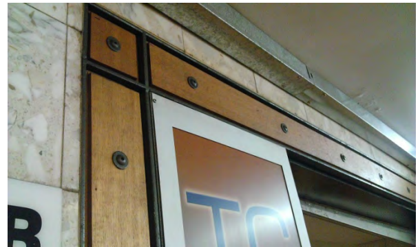
Figure 3.25 Detail of timber and metal surrounds to shopfronts in the Wynyard Station pedestrian arcades. This same treatment appears in the Menzies arcade. (Source: GML 2014)
