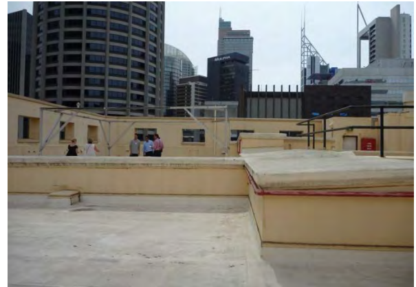
Figure 3.11 Roof terrace of the former Shell House, showing the high parapet with original openings. (Source: GML 2014)
