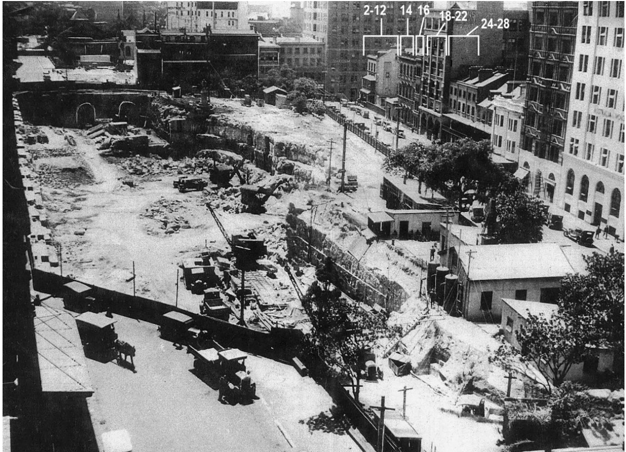
Figure 2.26 c1927 photograph looking north showing the excavation of Wynyard Park for the construction of the underground platforms and tunnels for Wynyard Station. This image was taken just prior to the demolition of the buildings numbered 14–28 Carrington Street. (Source: State Library of NSW)
