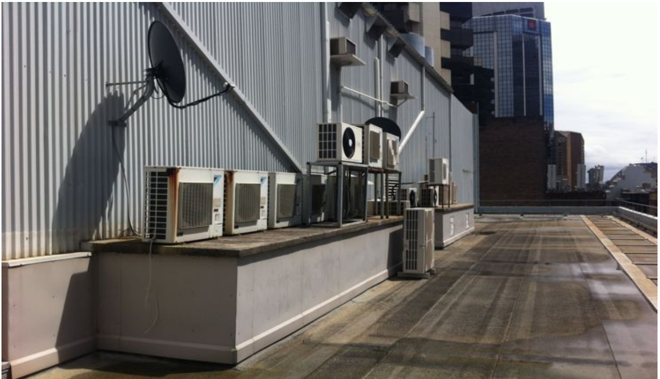
Photo 55: SMF waterproofing and air conditioning units containing SMF insulation on the Rooftop Level of 301 George Street, Sydney.
