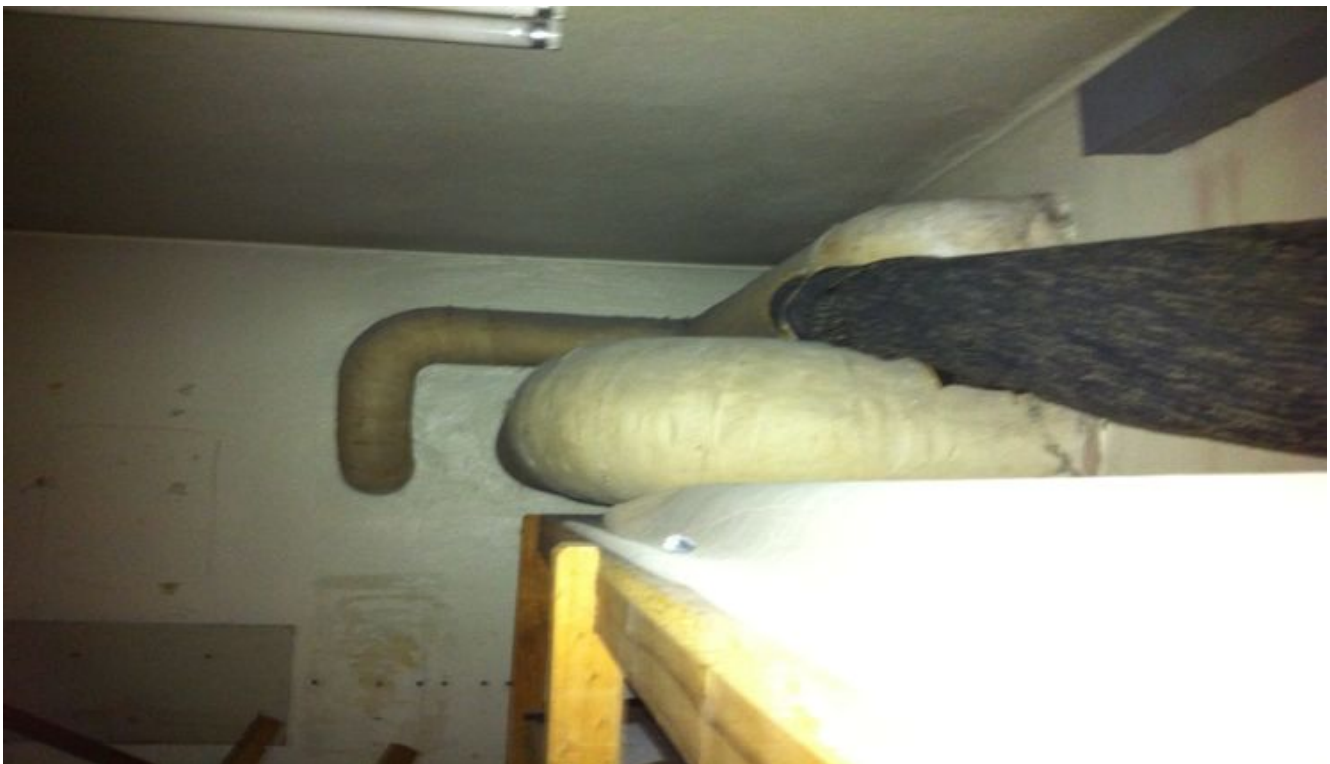
Photo 24: Asbestos insulated pipe work in the Store Room on Level 4 of the South Wing – Menzies Hotel.
