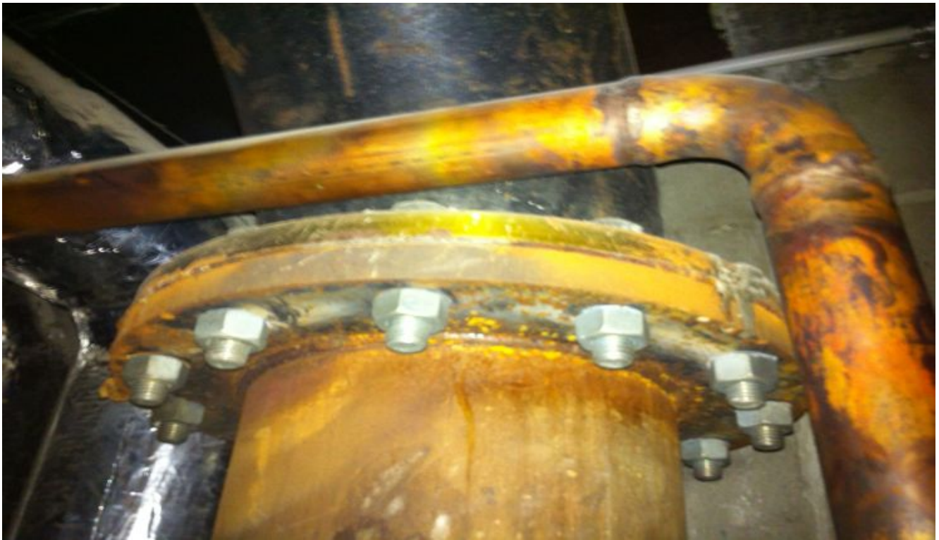
Photo 41: One (1) asbestos gasket on the large copper pipe work within the Main Western Riser on Level 3 of 301 George Street, Sydney.
