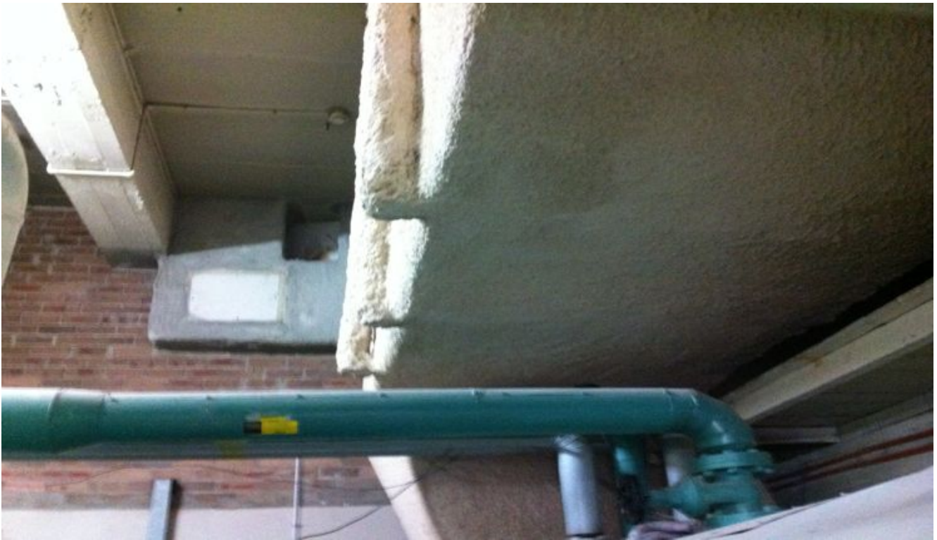
Photo 51: Sprayed SMF insulation located within Plant Rooms throughout the South Wing – Menzies Hotel.
