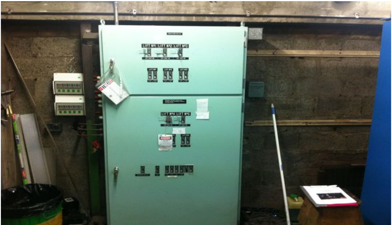
Photo 39: One (1) electrical switchboard containing asbestos arc shields within the Lift Motor Room on Level 15 – 301 George Street, Sydney.
