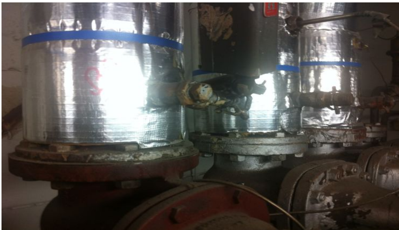
Photo 30: Hot water pipe work gaskets located within the Boiler Room on the Basement Level of the South Wing – Menzies Hotel.
