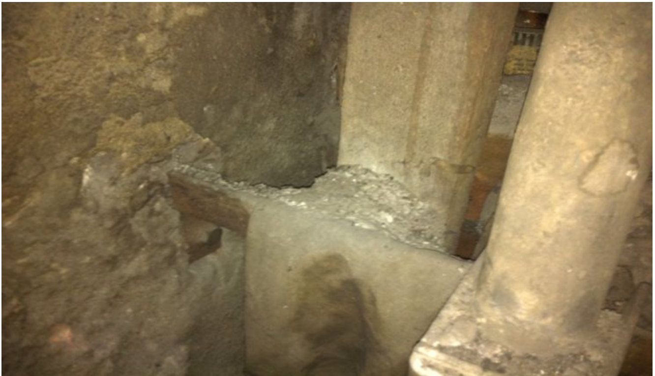
Photo 35: Asbestos lagging debris located within the Plumbers Riser Cupboard adjacent to the Entrance of the Wynyard Lane Car Park.
