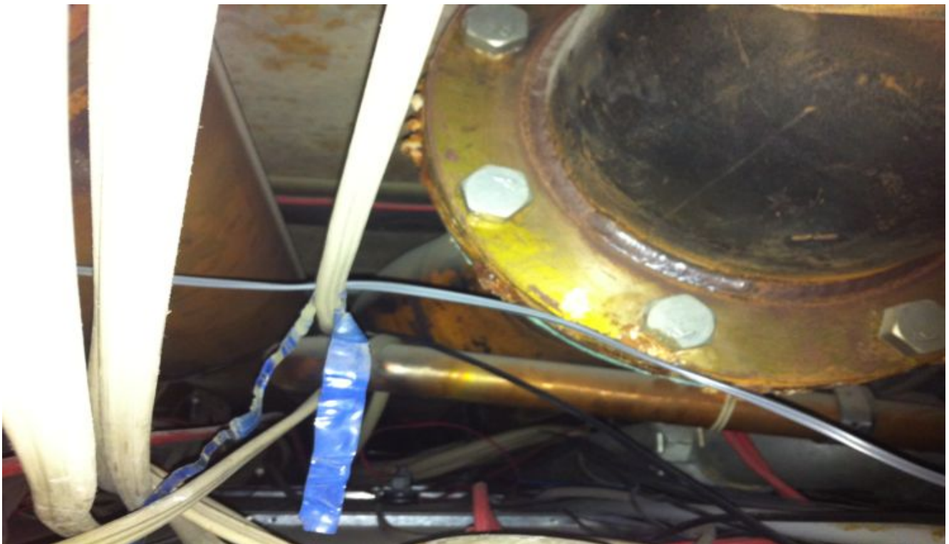
Photo 42: One (1) asbestos gasket on the large copper pipe work within the ceiling space of the Main Hallway on Level 2 of 301 George Street, Sydney
