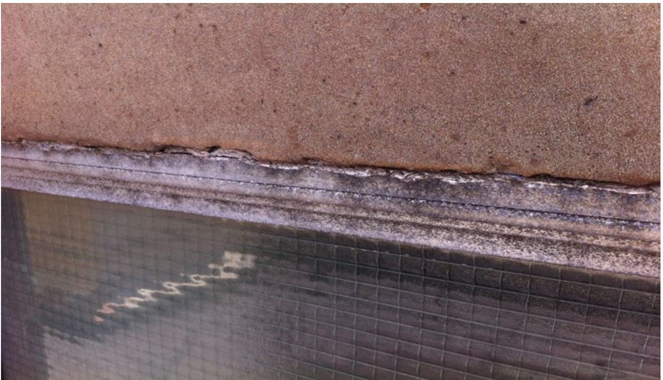
Photo 12: Mastic containing asbestos on the external window frames on Level 16 of South Wing – Menzies Hotel.
