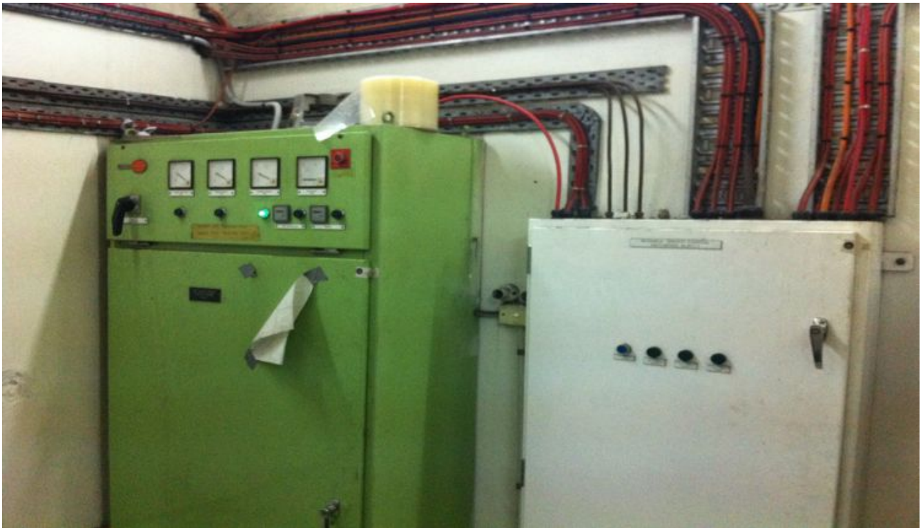
Photo 5: Two (2) electrical switchboards located within the Air Supply/Exhaust Plant Room on the Rooftop Level of the North Wing – Menzies Hotel.
