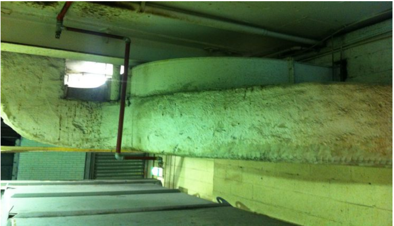
Photo 59: SMF insulation on the ductwork within the Loading Dock of 301 George Street, Sydney.
