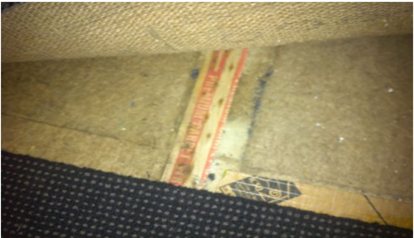
Photo 40: Vinyl floor tiles containing asbestos beneath the carpet on all Tenanted Levels of 301 George Street, Sydney.
