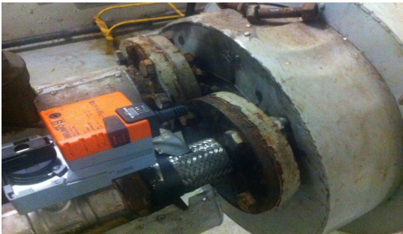
Photo 18: Asbestos gaskets located in the Plant Room on Level 15 of the South Wing – Menzies Hotel.
