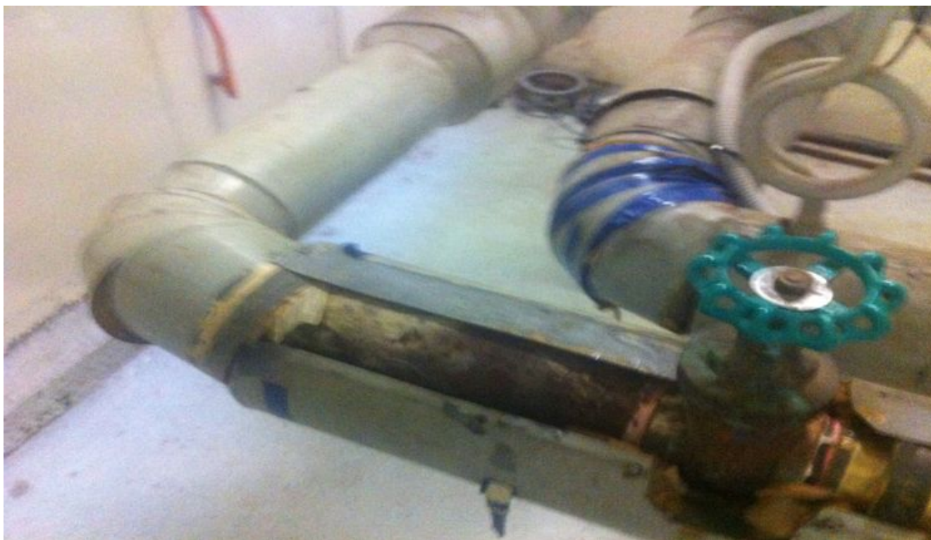
Photo 50: Pipe work containing SMF insulation throughout the Plant Rooms within the South Wing – Menzies Hotel.
