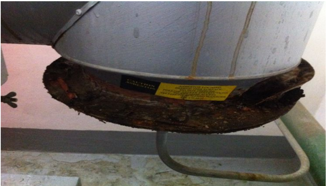
Photo 6: One (1) gasket containing asbestos located at the back of the boiler within the Boiler Room on the Rooftop Level of the North Wing – Menzies Hotel.
