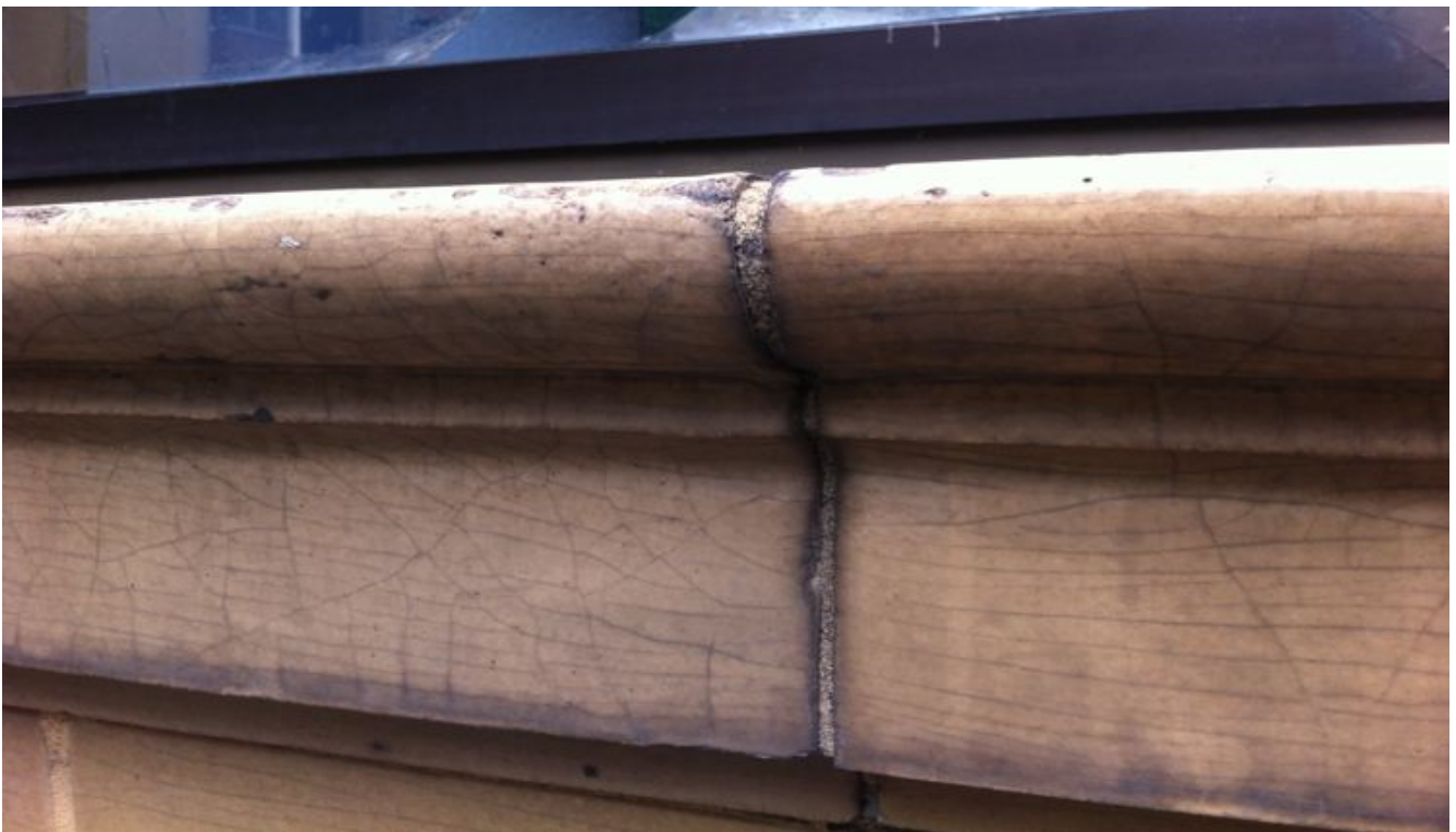
Photo 2: Caulking containing asbestos on the external façade to the North Wing – Menzies Hotel.
