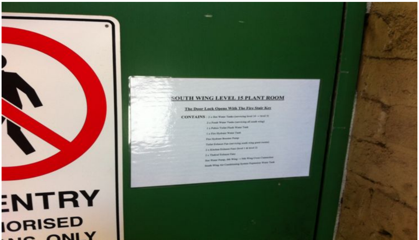
Photo 16: A sample of a Fire Door assumed to contain asbestos core throughout the South Wing – Menzies Hotel.
