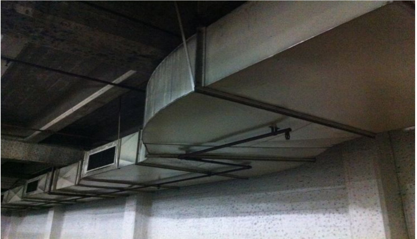
Photo 53: Ductwork containing internal SMF insulation located throughout the Wynyard Lane Car Park.
