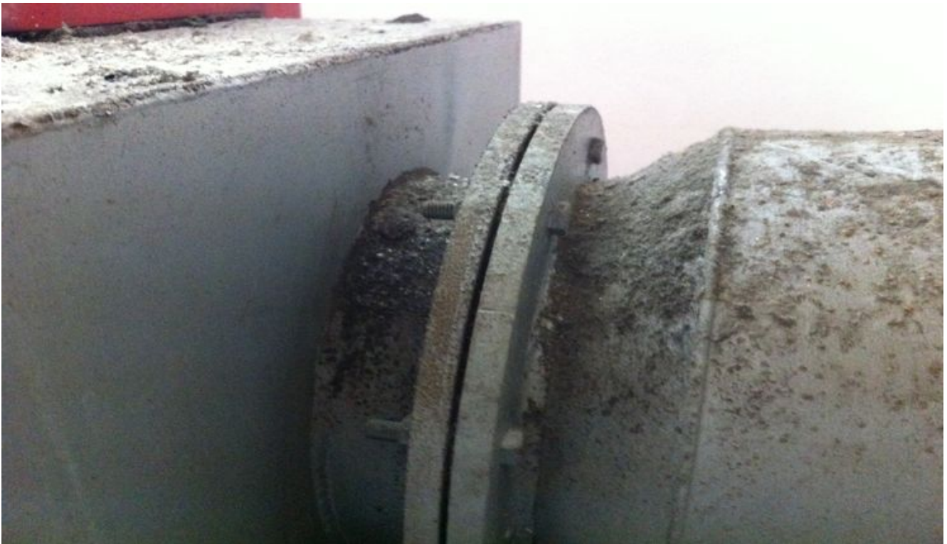
Photo 7: One (1) rope flange containing asbestos on the boiler within the Boiler Room on the Rooftop Level of the North Wing – Menzies Hotel.
