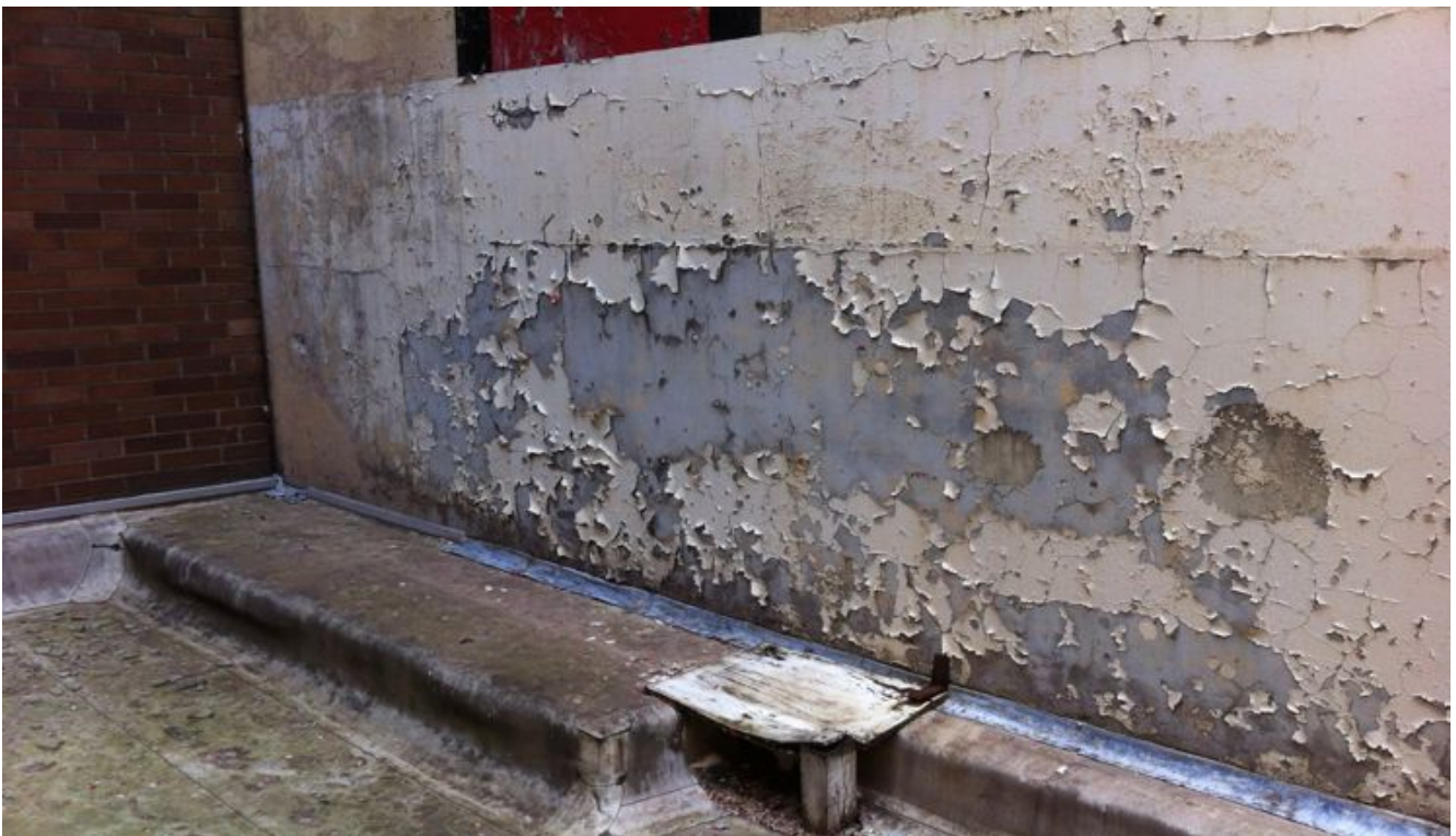
Photo 46: Beige paint containing elevated levels of lead on the external walls of Level 3 ½ on the South Wing – Menzies Hotel.
