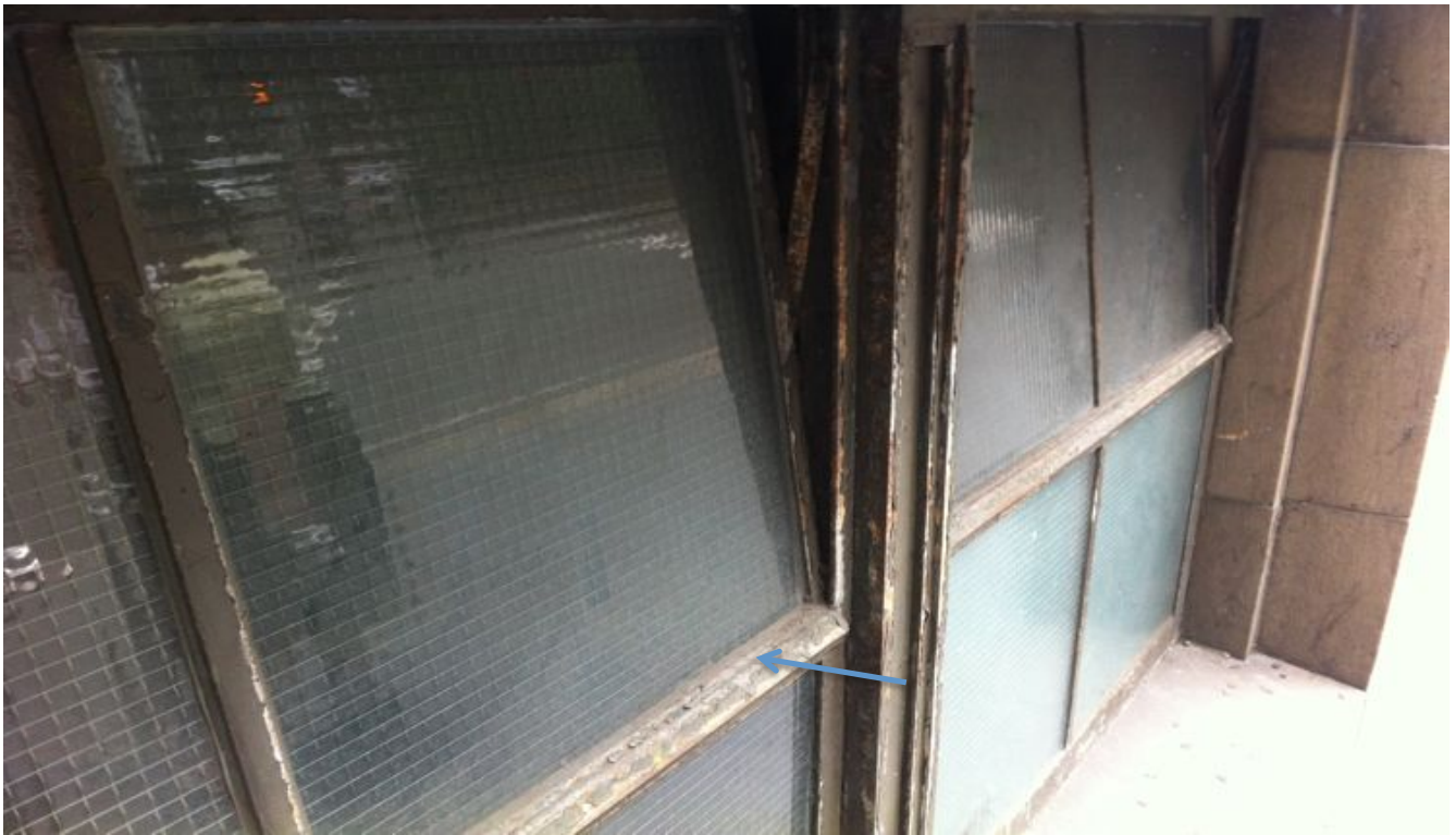
Photo 3: Window mastic containing asbestos on the external window frames of the North Wing – Menzies Hotel.
