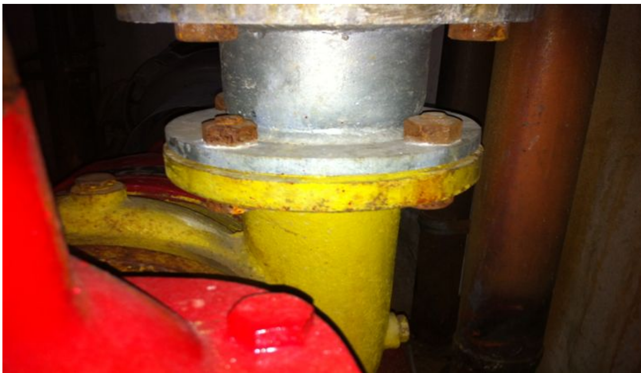
Photo 47: Yellow paint containing elevated levels of lead on pipe work within the Hydrant Booster Pump Room on Level 3 of 301 George Street, Sydney.
