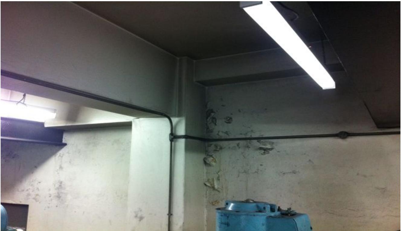
Photo 45: Beige paint containing elevated levels of lead on the ceiling and walls within the Lift Motor Room on the North Wing – Menzies Hotel.
