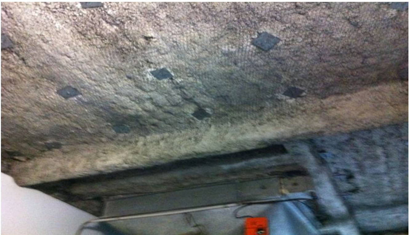
Photo 56: SMF insulation on the ceiling of the Fire Stairwell of 301 George Street, Sydney.
