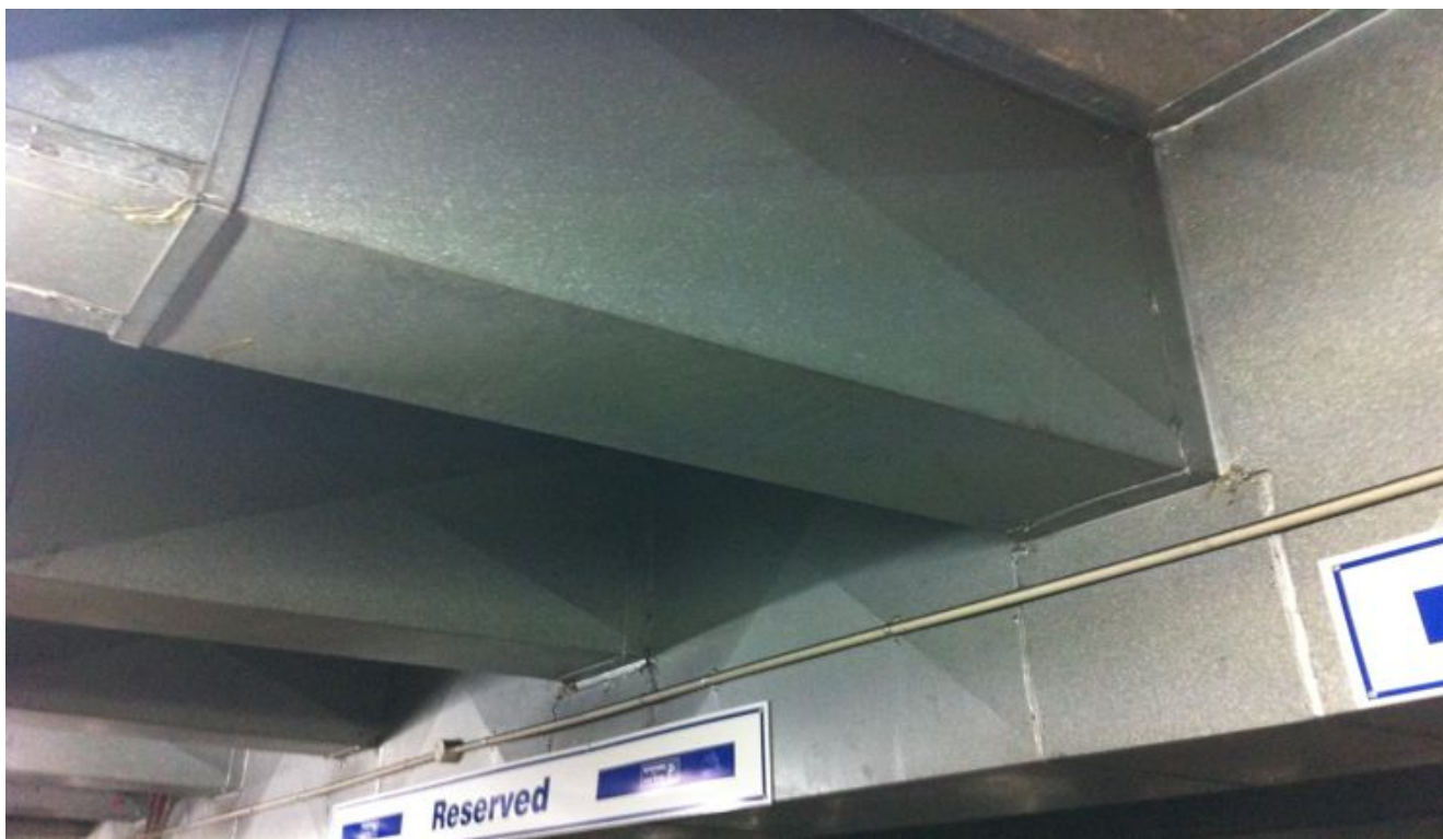
Photo 31: Encapsulated ceilings containing asbestos lagging insulation located throughout the Upper Tunnel of the Wynyard Lane Car Park.
