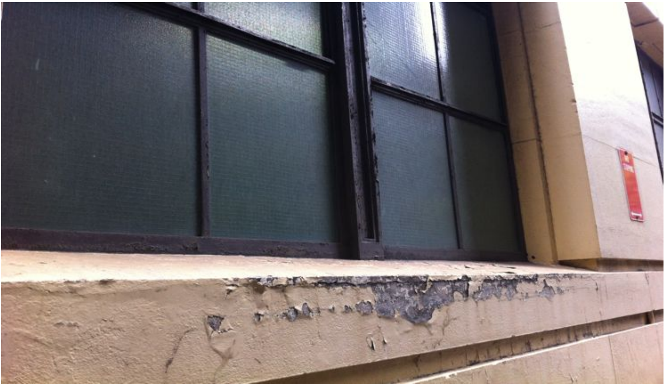
Photo 43: Brown and yellow paint containing elevated levels of lead on the external area of the North Wing – Menzies Hotel.
