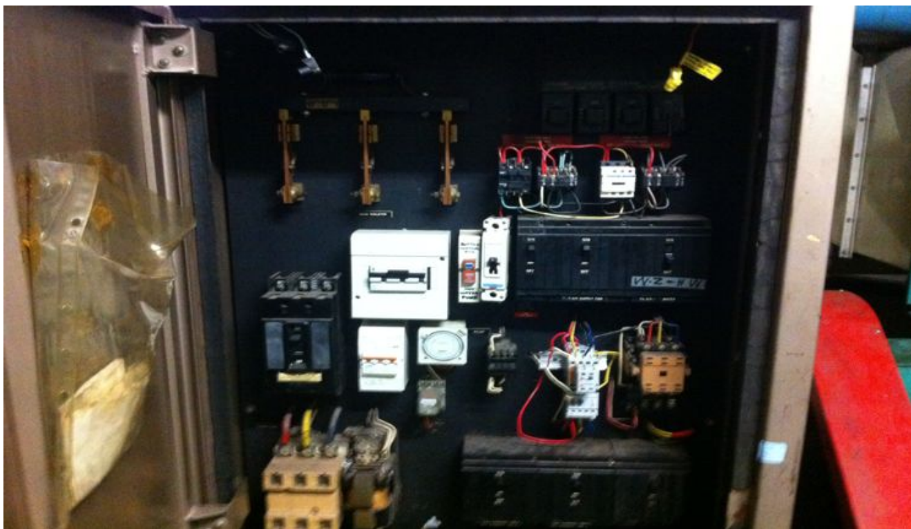
Photo 19: One (1) of two (2) bituminous backing boards containing asbestos adjacent the entrance door to the Plant Room on Level 15 of the South Wing – Menzies Hotel.
