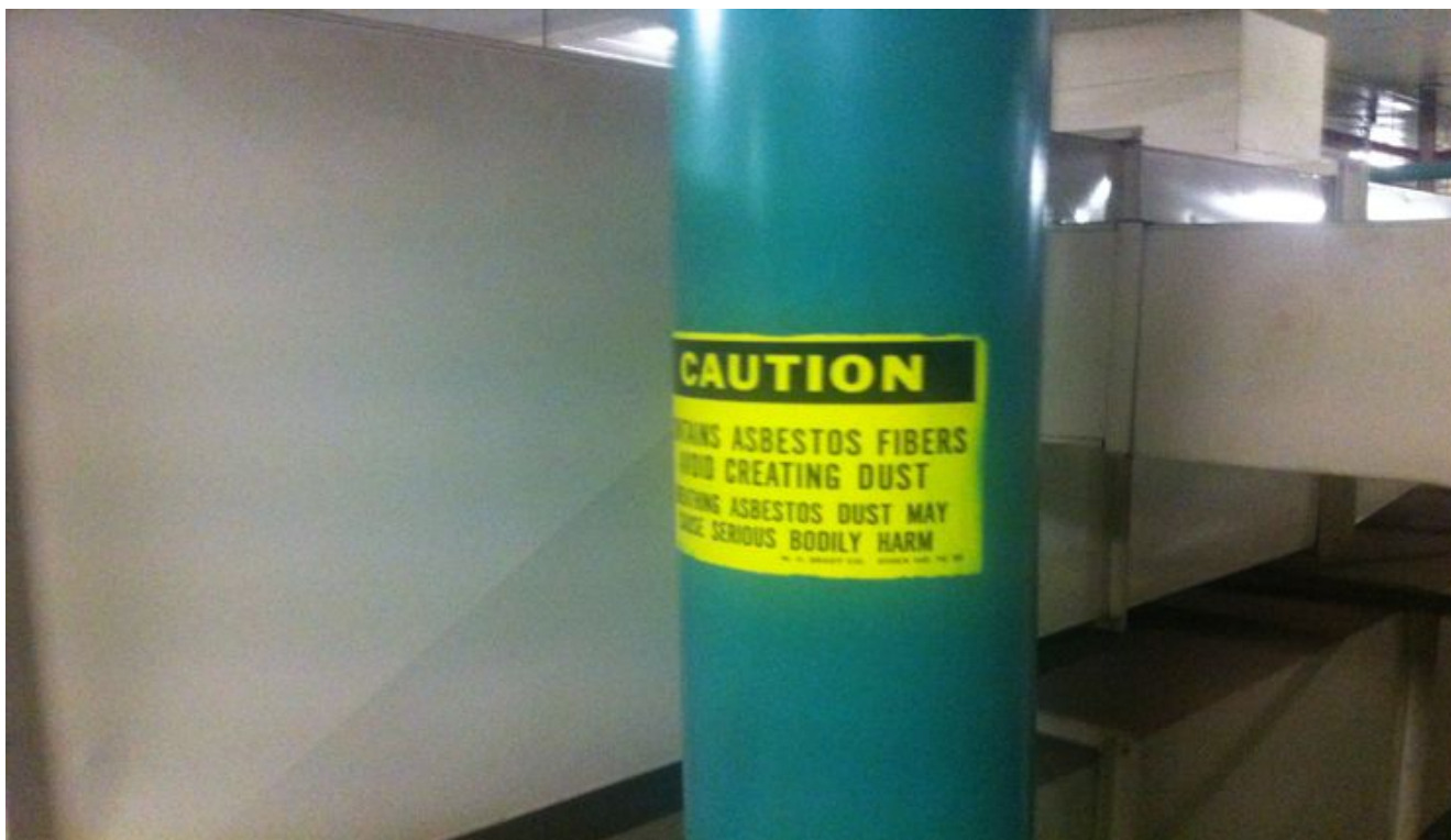
Photo 17: Pipe work containing asbestos insulation located throughout the Plant Room on Level 15 of the South Wing – Menzies Hotel.
