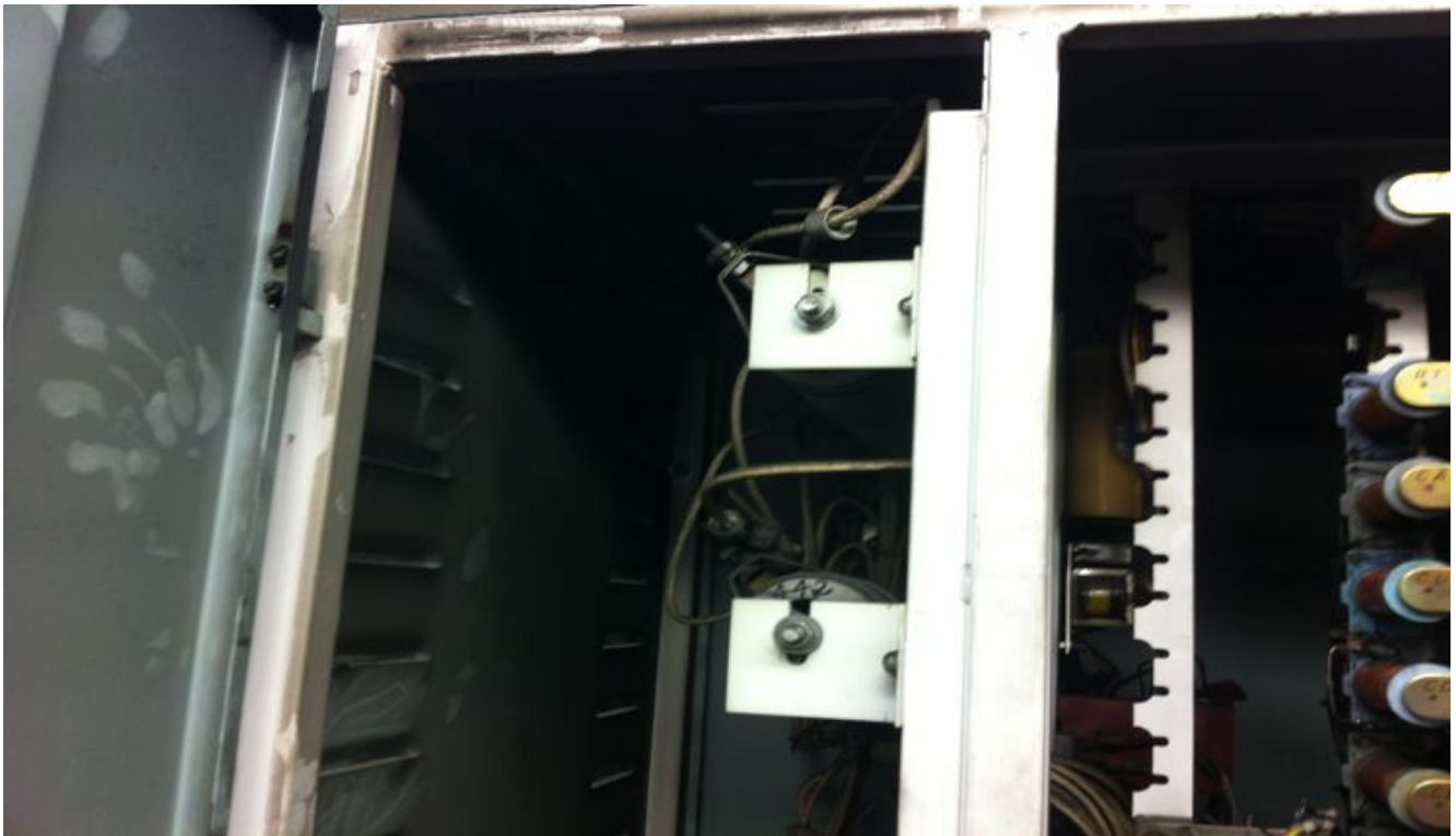
Photo 9: Cable insulation containing asbestos within the Control Cabinets of the Lift Motor Room of the North Wing – Menzies Hotel.
