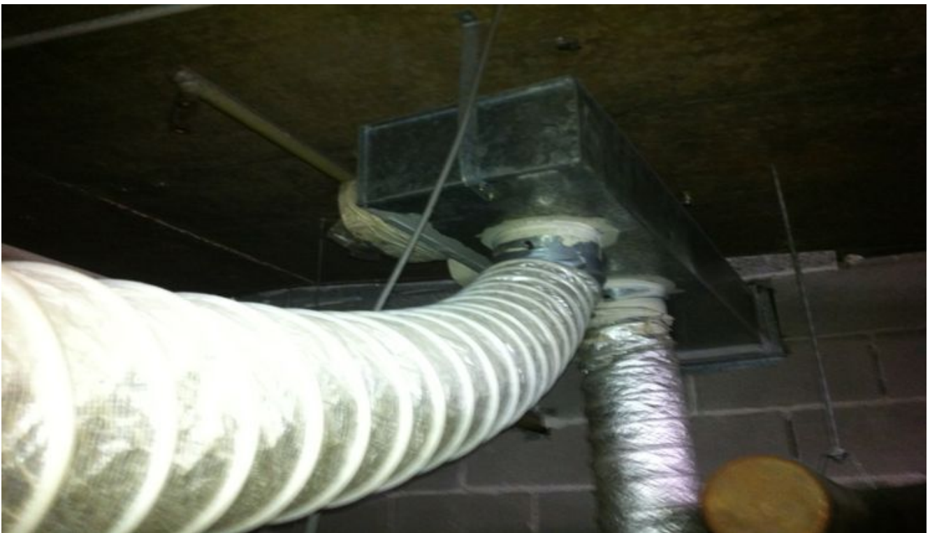
Photo 60: SMF insulation within the air conditioning ductwork of the Retail Areas of 301 George Street, Sydney.
