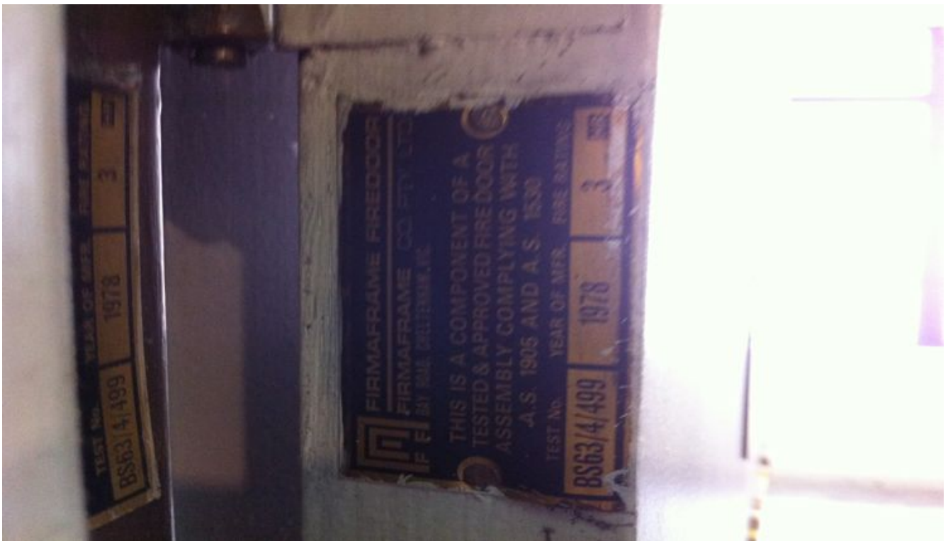
Photo 4: A sample of a Fire Door assumed to contain asbestos core throughout the North Wing – Menzies Hotel.
