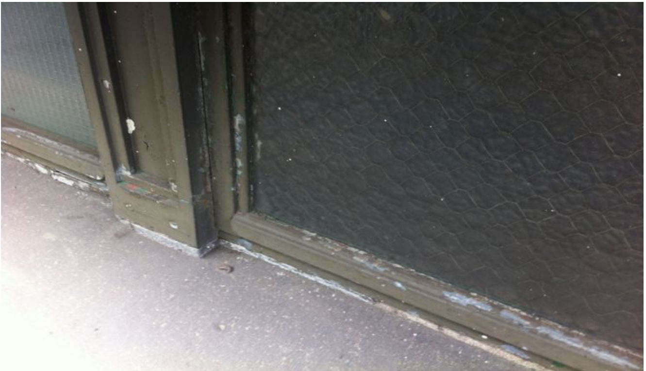
Photo 44: Green paint containing elevated levels of lead on the external window frames of the North Wing – Menzies Hotel.
