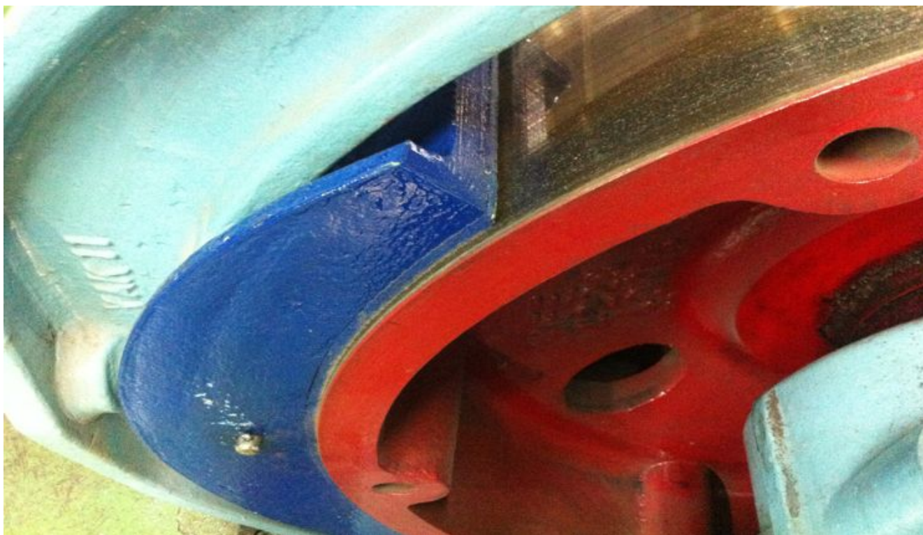
Photo 38: Bituminous brake pads containing asbestos on the Lift Motors located within the Lift Motor Room on Level 15 – 301 George Street, Sydney.
