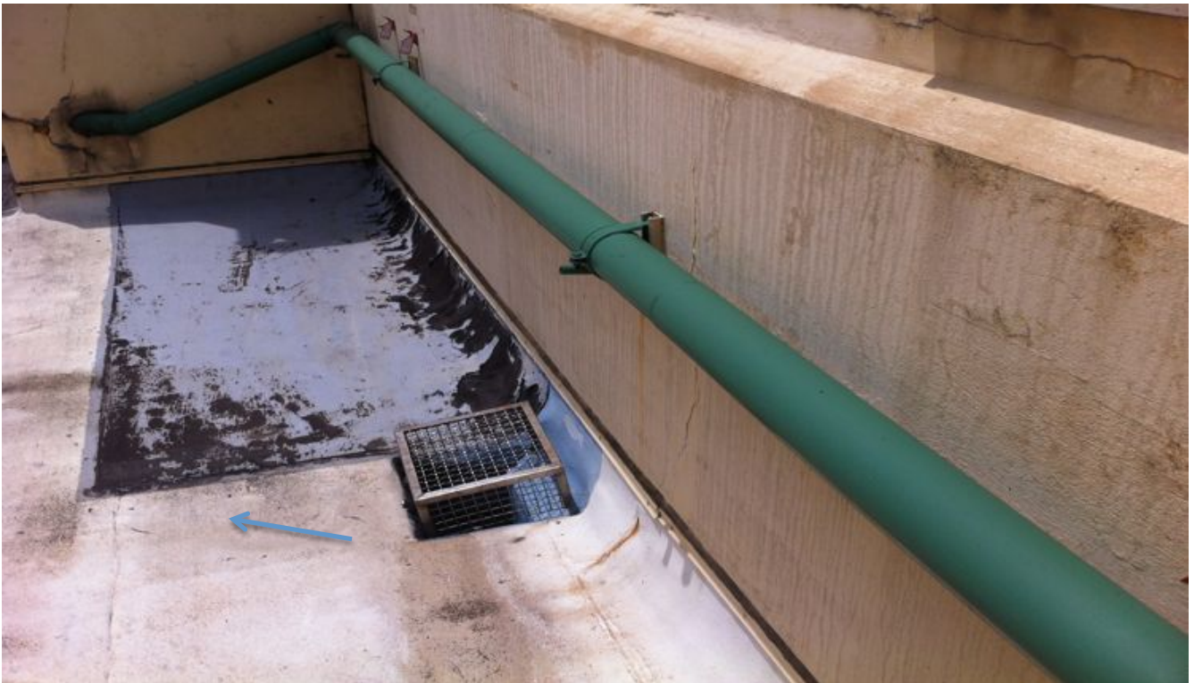
Photo 1: Bituminous waterproofing membrane containing asbestos and pipe work containing internal SMF insulation on the North Wing Rooftop Level – Menzies Hotel.
