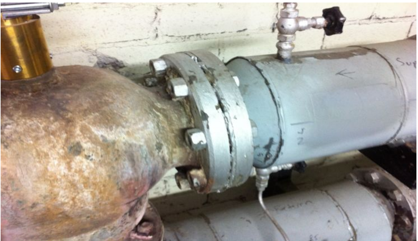
Photo 26: Asbestos gaskets in the Plant Room on Level 3 ½ of the South Wing – Menzies Hotel.
