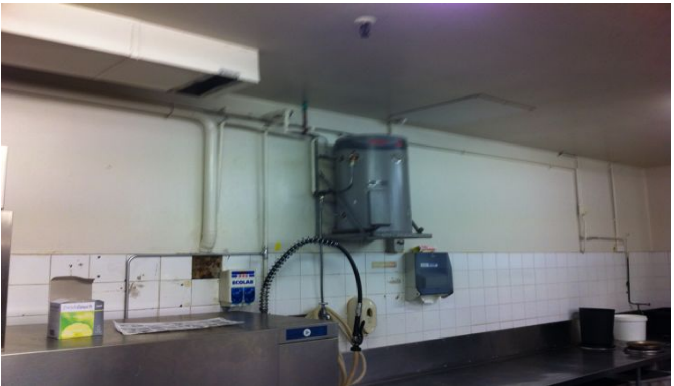
Photo 52: Various hot water systems containing internal SMF insulation located throughout the South Wing – Menzies Hotel.
