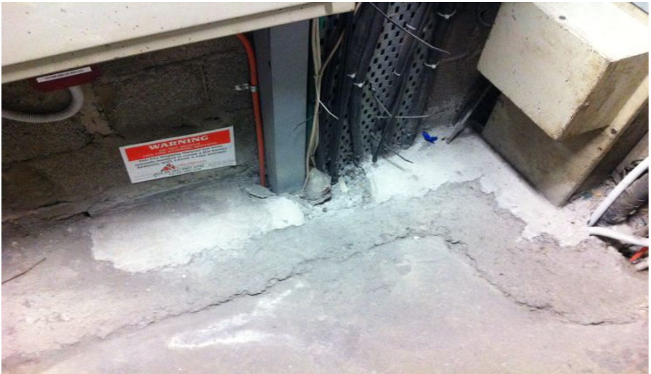
Photo 57: SMF fire rating in the penetrations within the riser cupboards of 301 George Street, Sydney.
