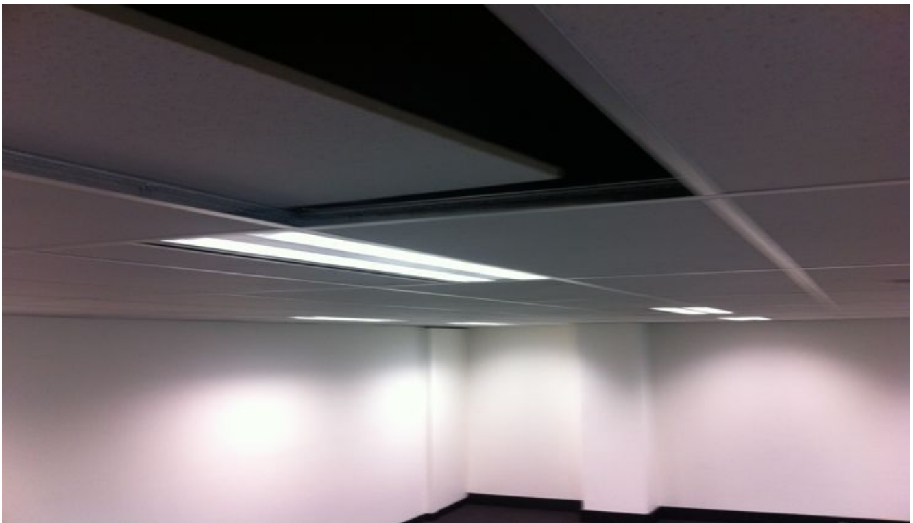
Photo 58: Cellulose ceiling tiles containing SMF within the Tenancies of 301 George Street, Sydney.
