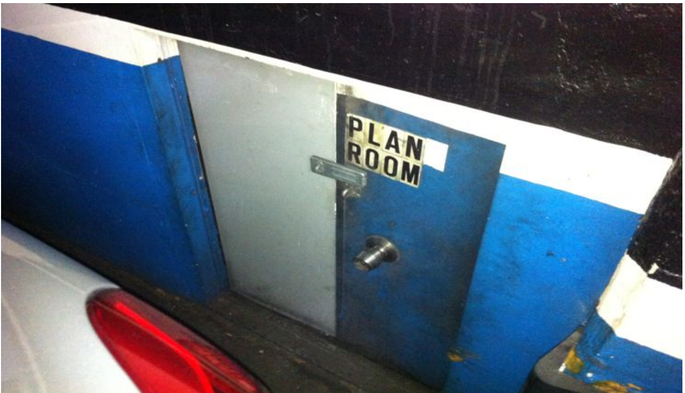
Photo 34: Fire doors containing asbestos on the Upper Level Plant Rooms of the Wynyard Lane Car Park.
