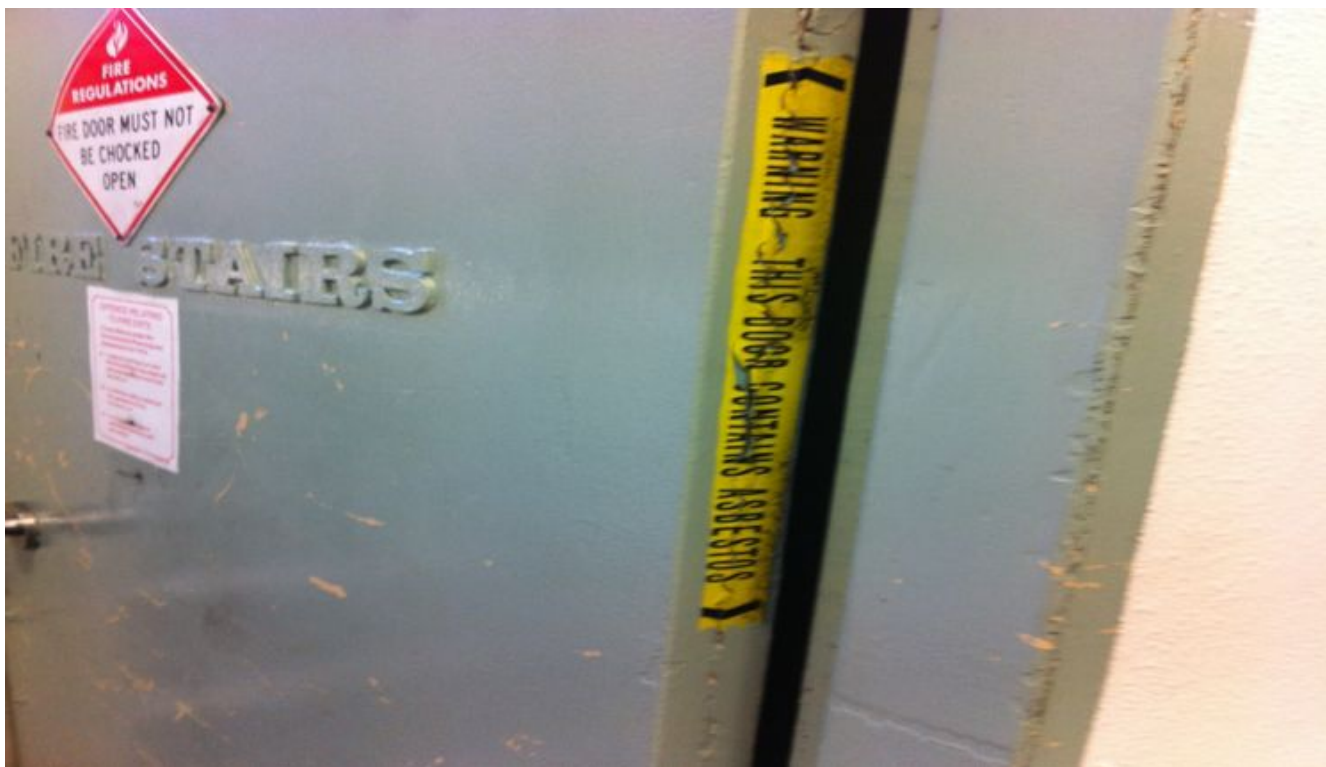
Photo 29: One (1) fire door containing asbestos from the Fire Stairs of the South Wing – Menzies Hotel.
