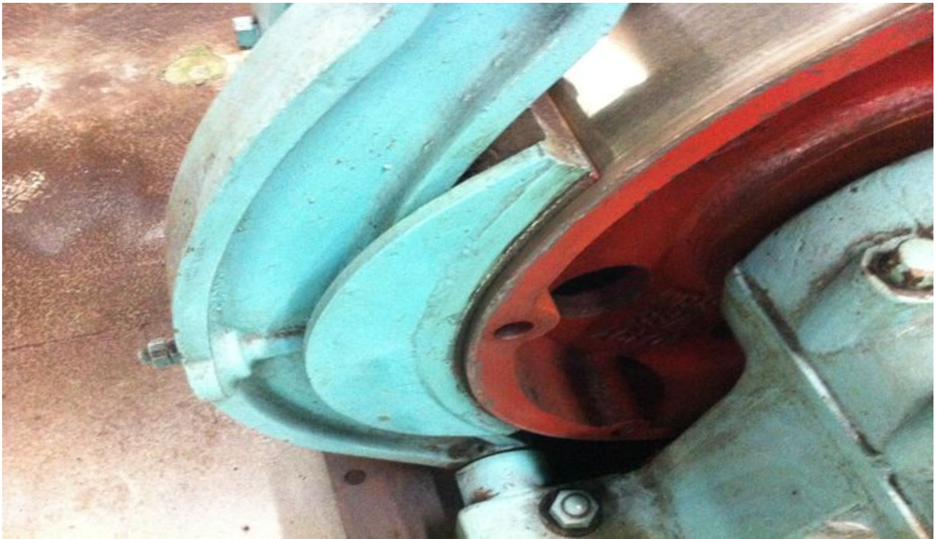
Photo 15: Bituminous brake pads assumed to contain asbestos within the Lift Motor Room of the South Wing – Menzies Hotel.
