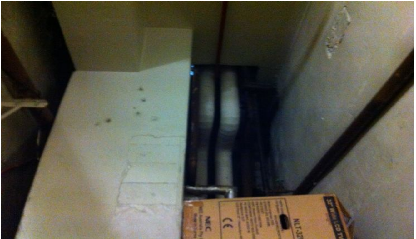
Photo 27: Two (2) large asbestos wrapped pipes within the AV Room of the Banquet Kitchen on Level 2 of the South Wing – Menzies Hotel.
