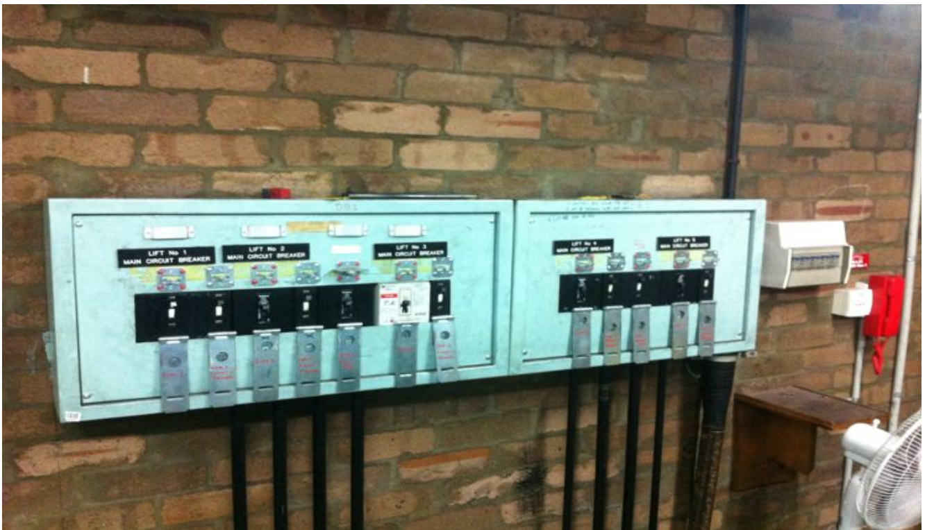
Photo 14: Two (2) electrical switchboards containing asbestos located within the Plant Room on the Lift Motor Room Level of the South Wing – Menzies Hotel.
