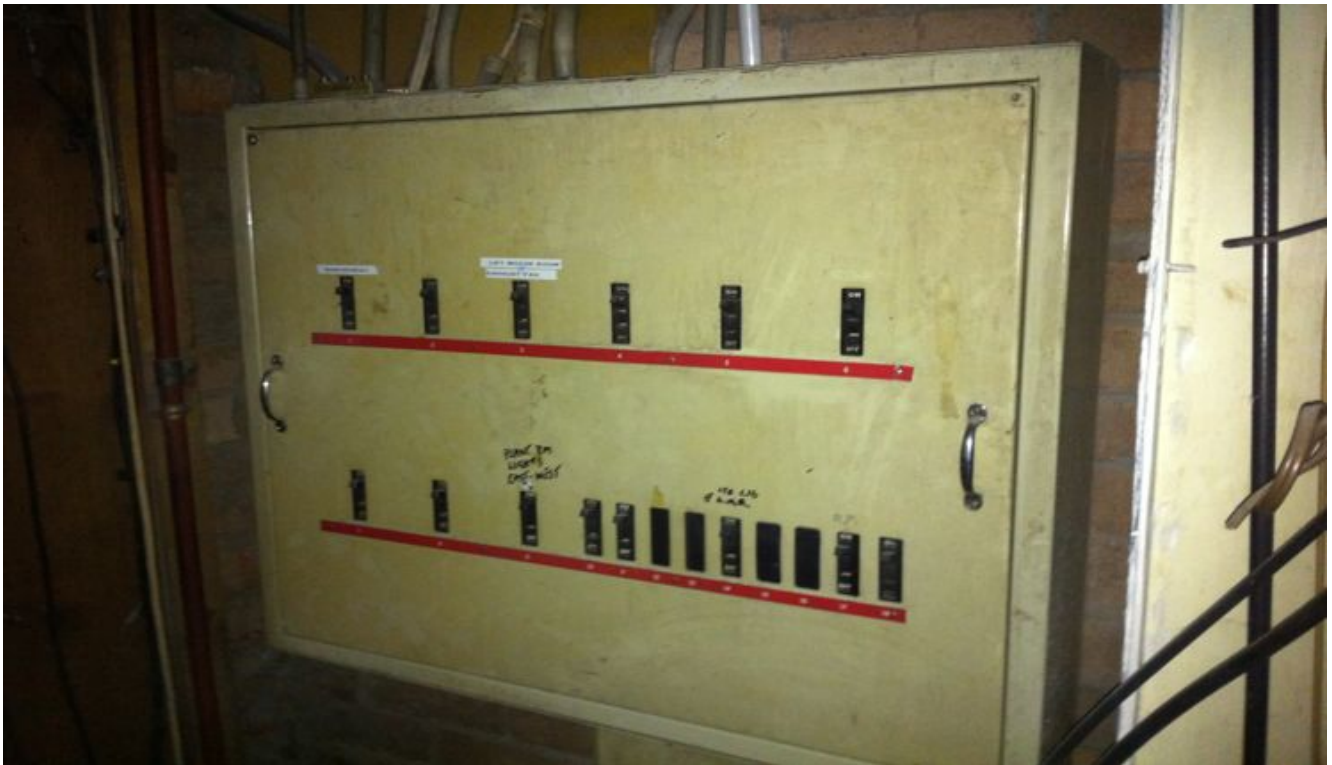
Photo 21: One (1) electrical distribution cupboard within the Lifties Room on Level 15 of the South Wing – Menzies Hotel.
