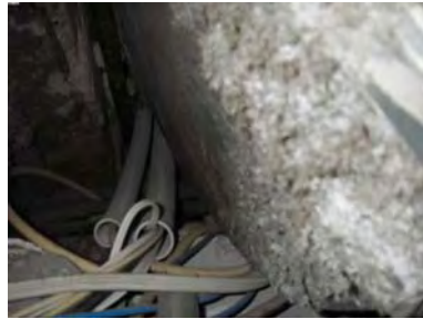
Photo 2. MW02 Main Hospital; Kitchen Lobby, Ceiling Space – Asbestos containing insulation
