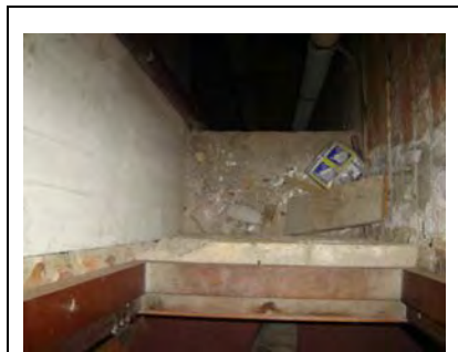
Photo 1. Asbestos containing pipe lagging debris within the pipe riser
