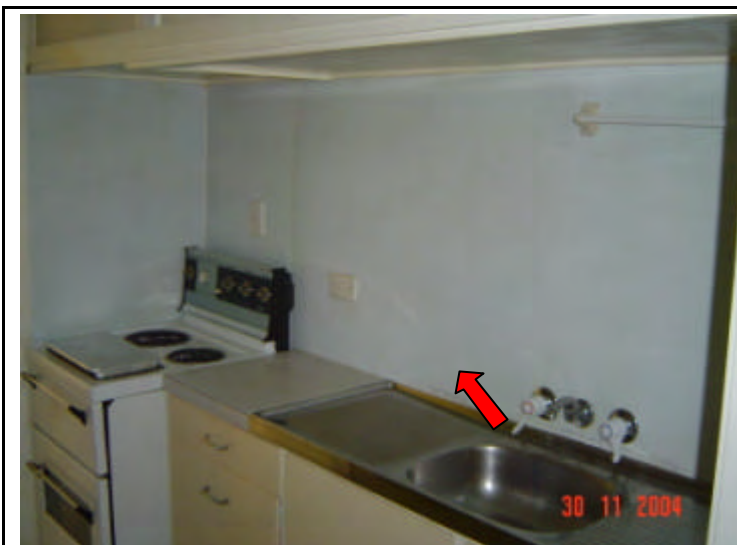
Photograph 1 : Kitchen, lower wall panelling behind stove and sink – showing asbestos-containing fibre-cement sheet panels
