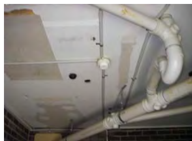
Photo 1. Asbestos soft board ceiling in Main Switchroom
