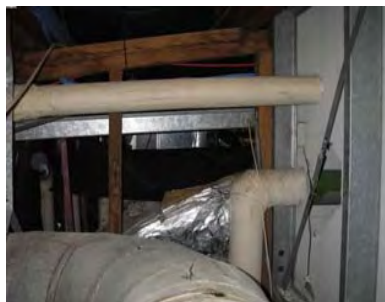
Photo 1. Asbestos containing pipe lagging within Hewitt Block
