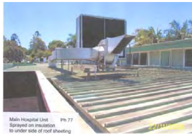
Photo 1. Asbestos sprayed insulation on underside of metal roof, Throughout ceiling space of Main Hospital (MU1)
