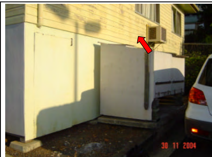
Photograph 1: E Block exterior, showing lead-containing horizontal wall panelling paint
