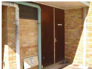
Photo 1. Asbestos containing fire doors at entrance of BB01 Operating Theatres
