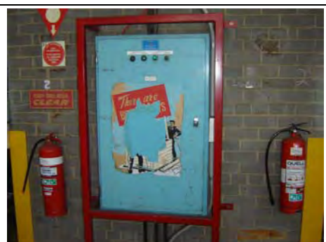
Photograph No.4: An example of a suspected asbestos containing electrical backing board
