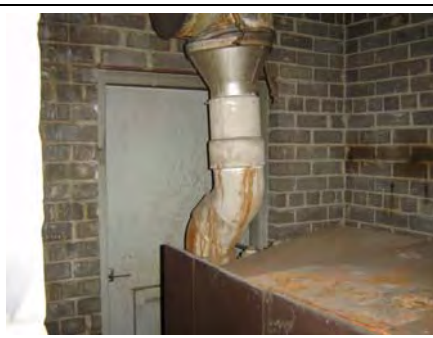
Photograph No.2: An example of an asbestos cement sheet boiler flue
