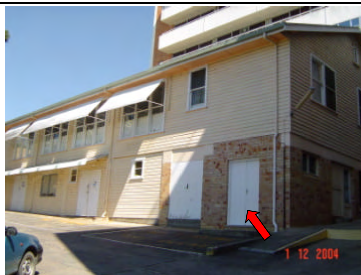
Photograph 2: G Block exterior – showing lead-containing paint on workshop entry doors
