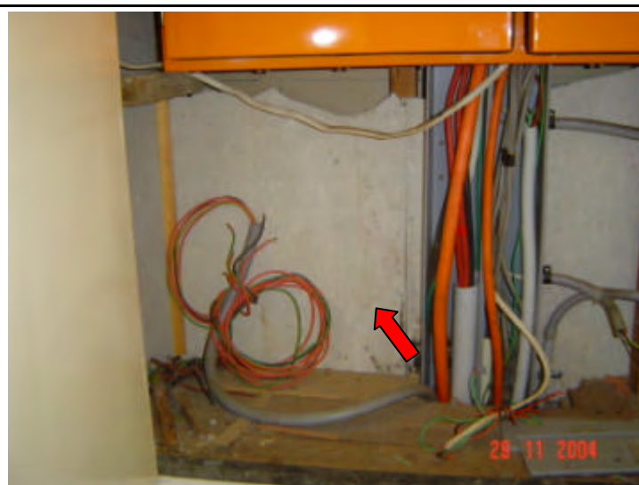
Photograph 2: E Block Level 1, Staff lounge – distribution board ward 9 cupboard – showing asbestos-containing wall panels
