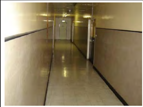
Photograph No. 5: An example of asbestos containing vinyl floor tiles
