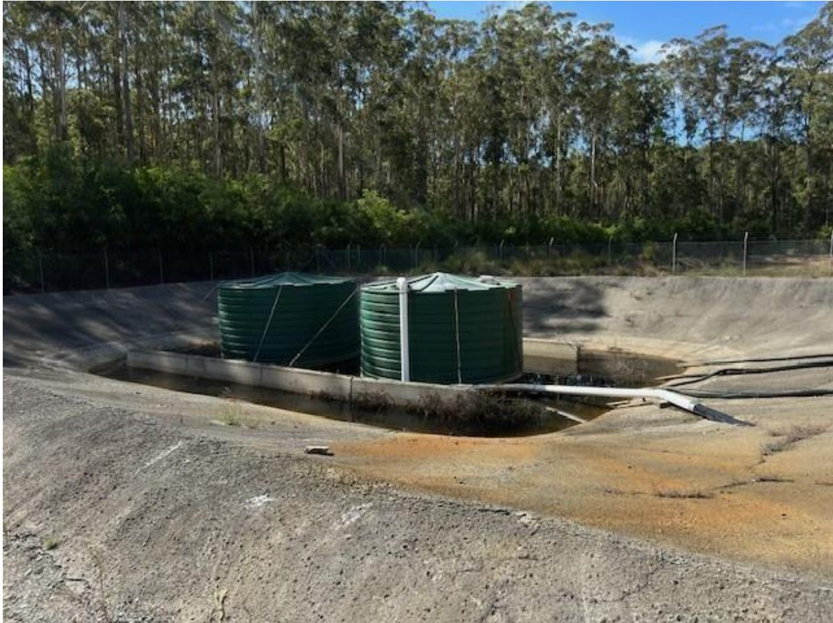
Bunded Above Ground Leachate Storage Tanks.
