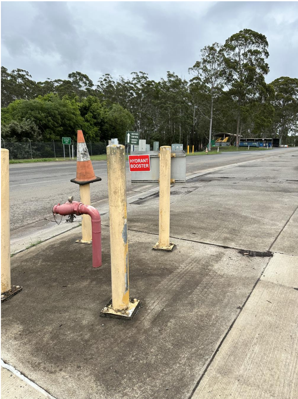
Fire hydrant booster
