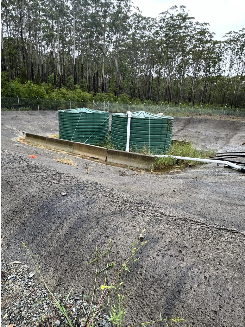
Bunded above ground leachate storage tanks
