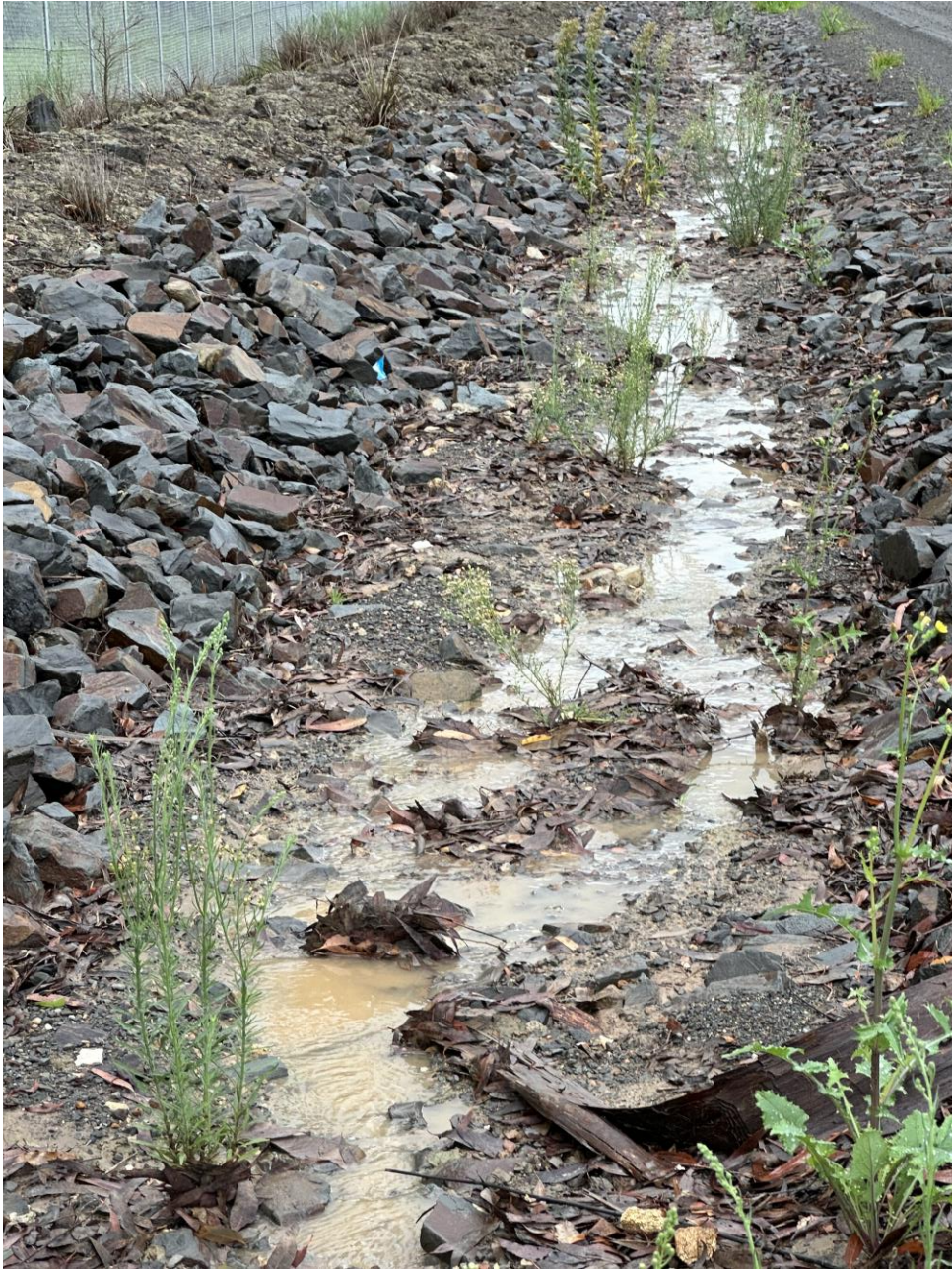
Diversion drains for clean stormwater
