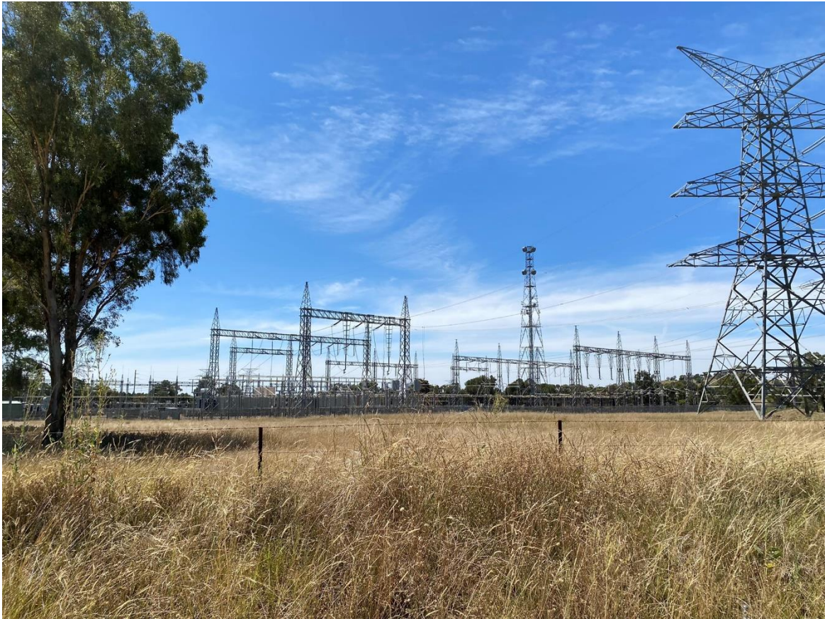
Plate 2-1: Transgrid Wagga Wagga 330kV substation
