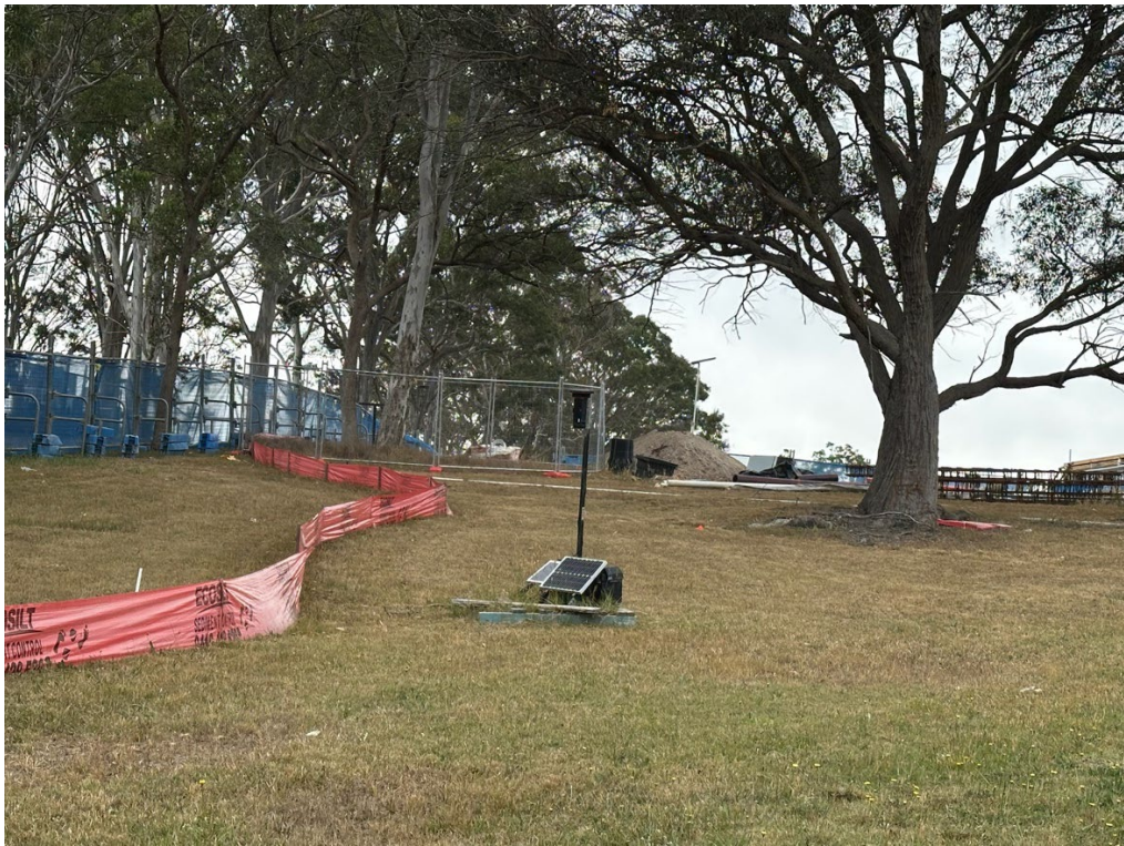
Photo 21: Realtime noise and dust monitor
