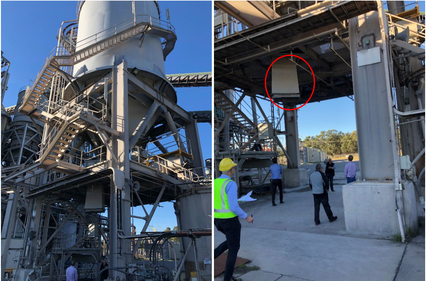
Figure 8.3. Photo of the existing ash storage silo (left), and overhead telescopic chute arrangement (right, circled in red) which enables ash to be discharged under gravity into a tanker truck for off-site transport.
