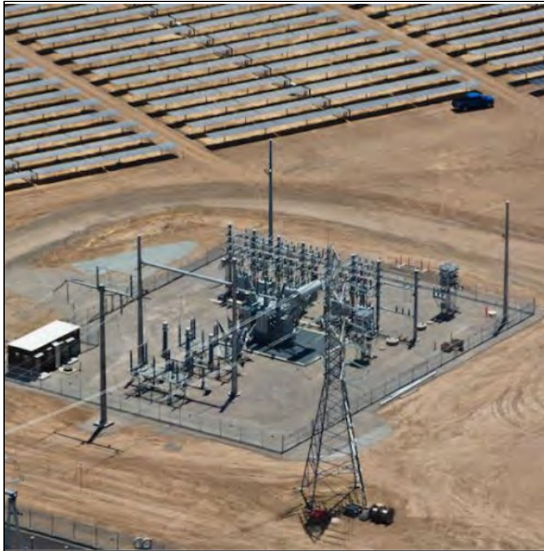
Plate 4-4: Typical Solar Farm Substation Footprint
