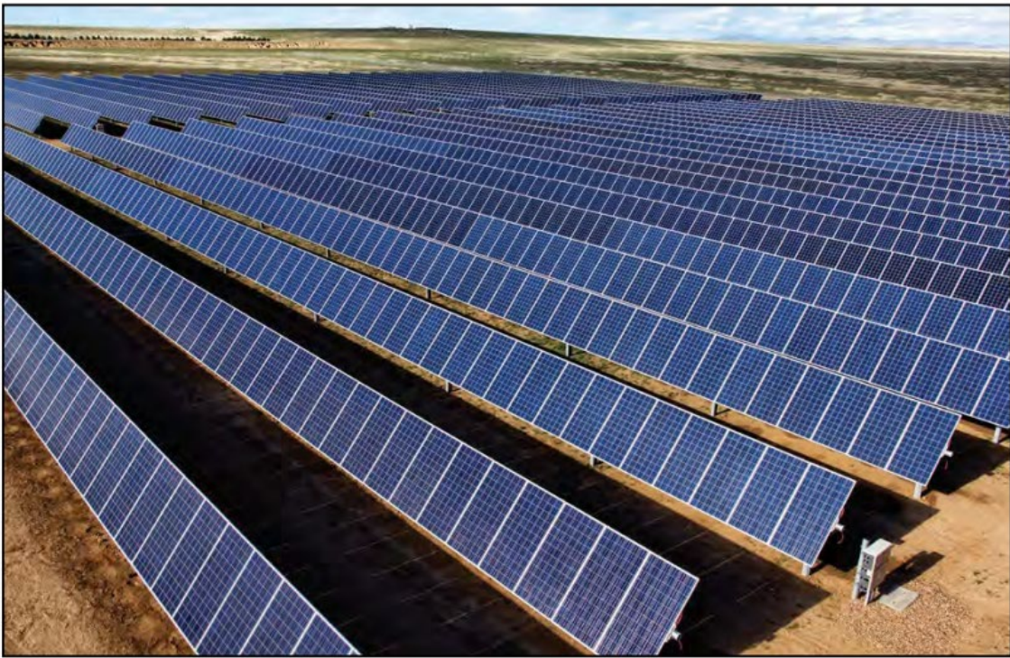
Plate 4-1: Typical Solar Panel Arrays
