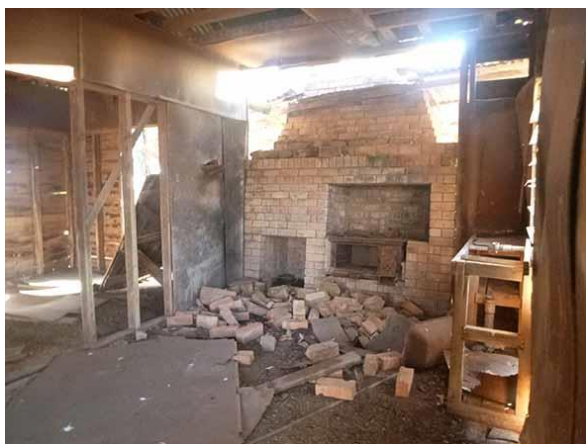
9. Double brick chimney with fireplace to the left and cast-iron oven to the right
