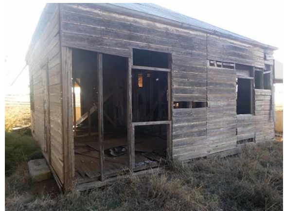
8. Eastern side of the dwelling with cladding removed exposing the hardwood timber frame.
