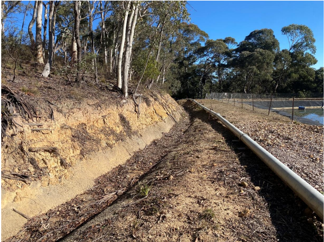
Photograph 25 – Clean water diversion drain
