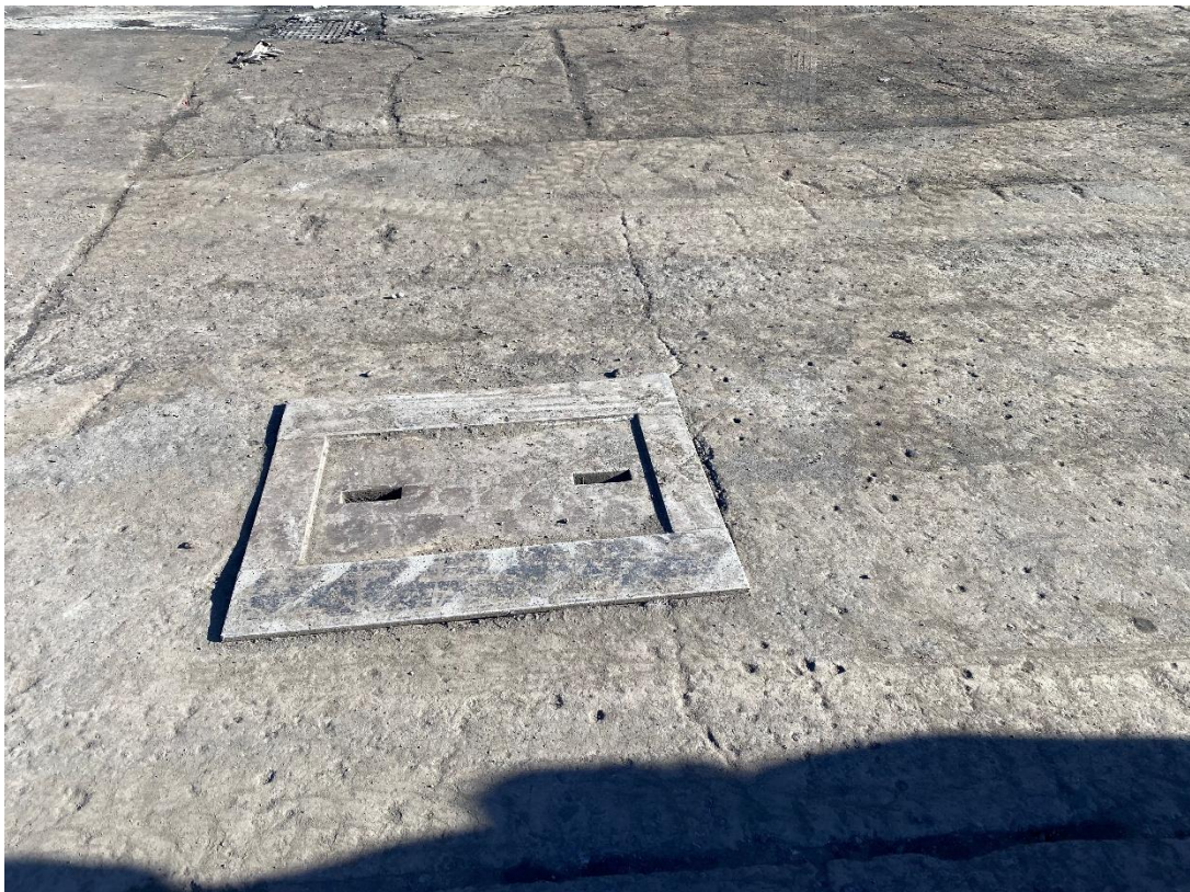
Photograph 34 – Oily water drain
