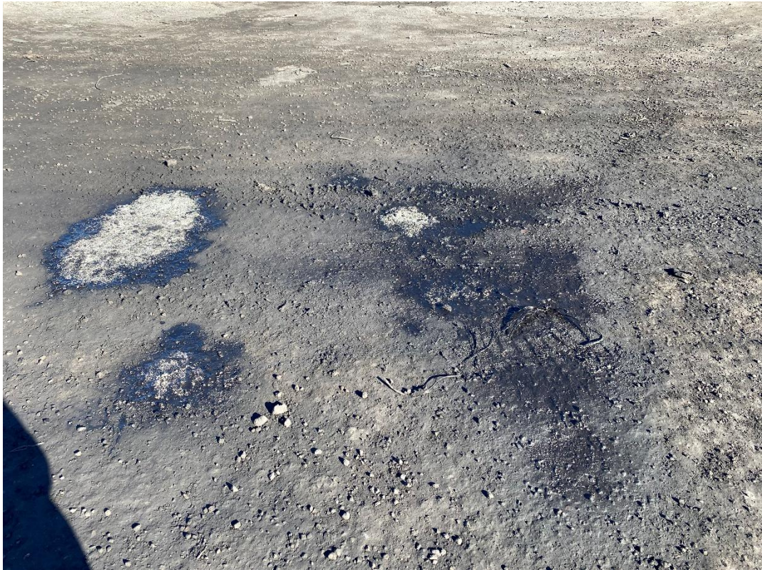
Photograph 31 – Recent hydrocarbon leak. Partially covered by sorb
