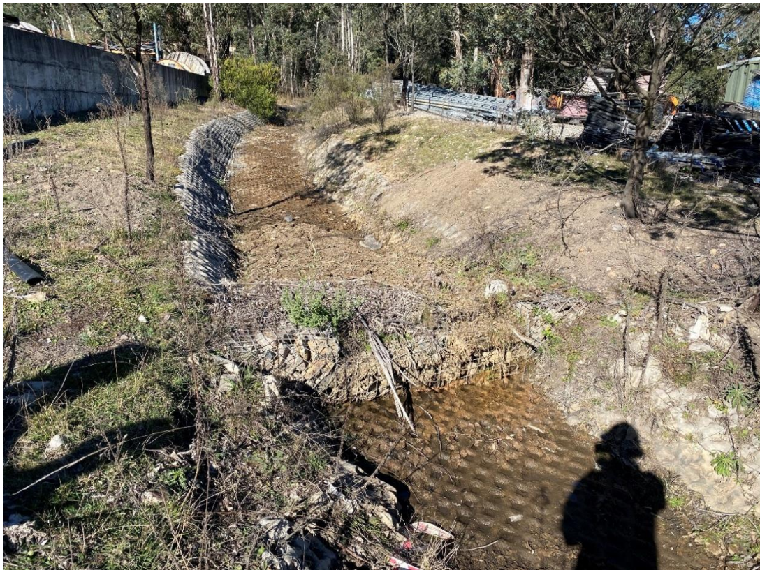
Photograph 20 – Sediment and debris to be removed from the transfer drain
