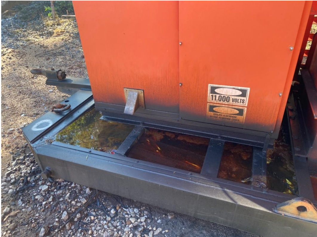
Photograph 21 – Leaks from old transformer
