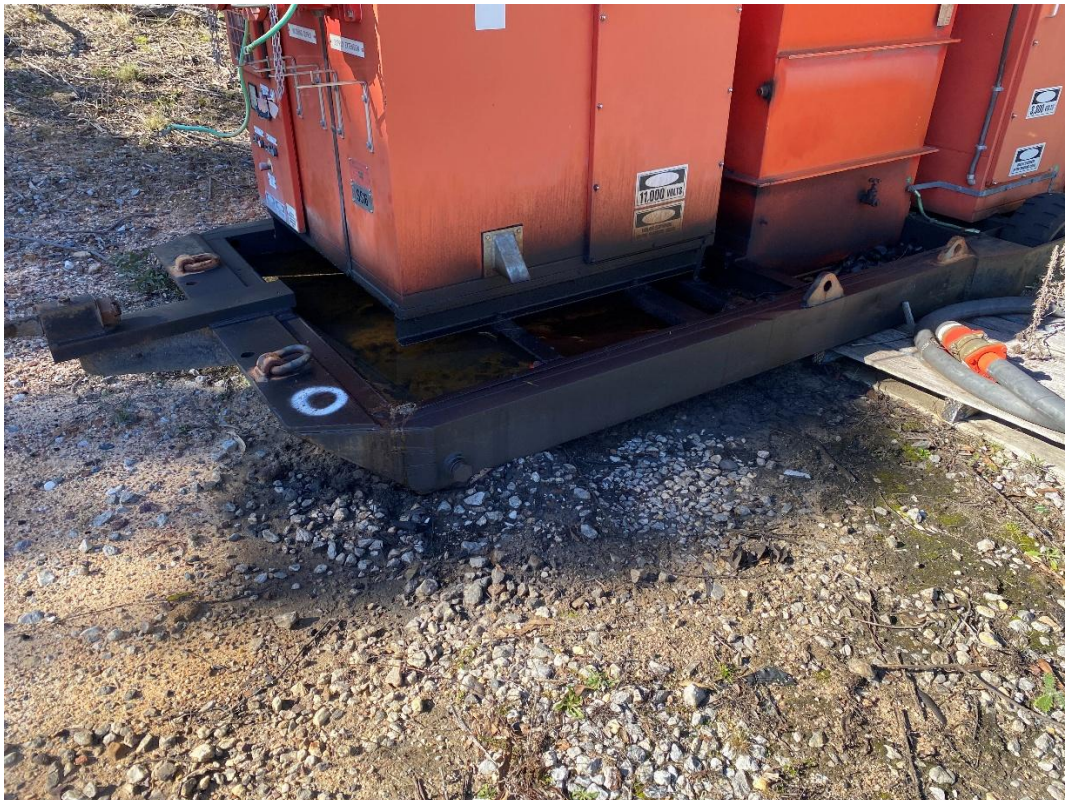
Photograph 22 – Evidence of hydrocarbon staining
