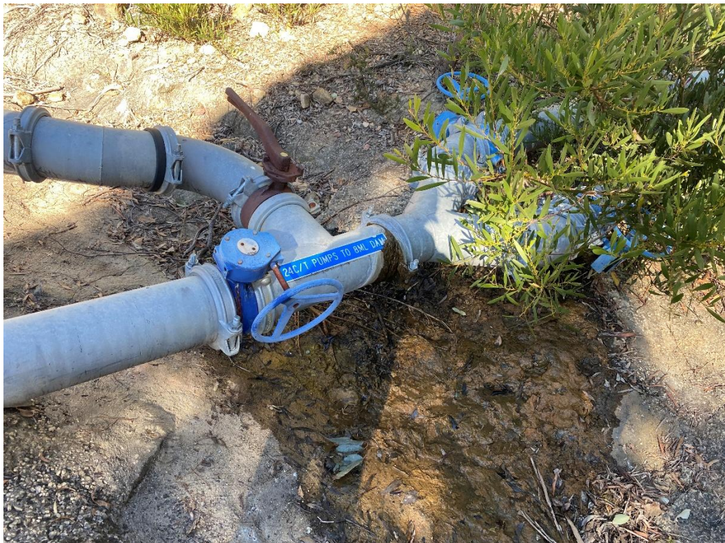
Photograph 26 – Pipeline leak to be repaired
