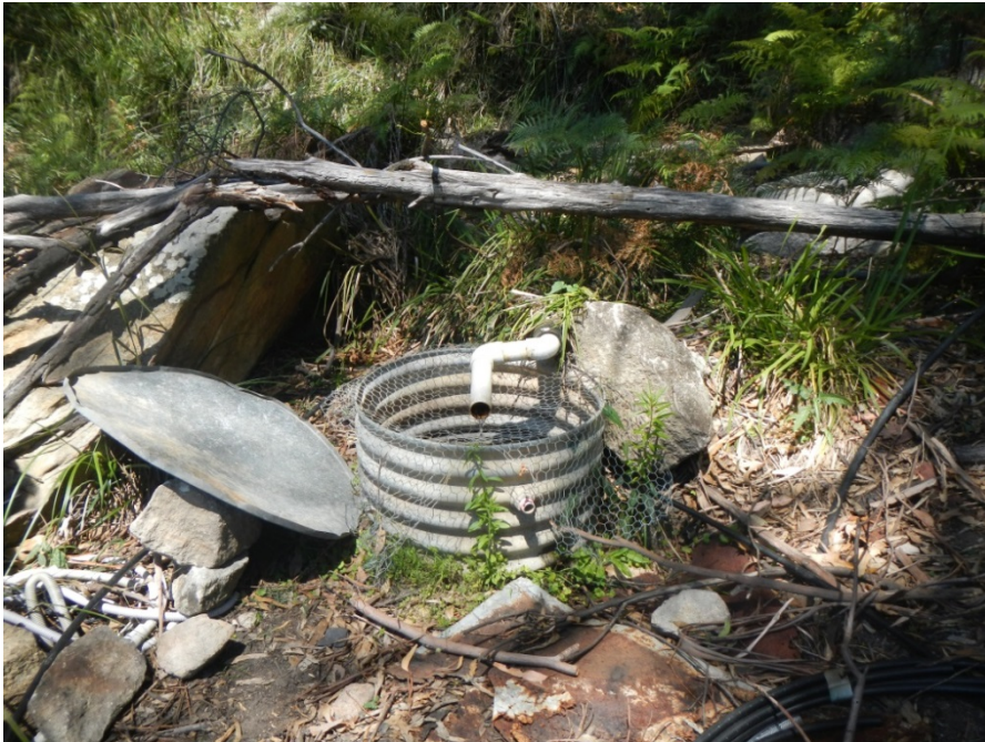
Figure 9: Airly Village spring (piped and usually covered).
