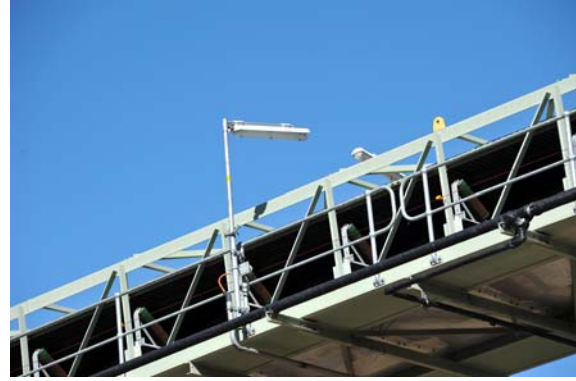
Plate 13 – Lighting on overhead conveyor
