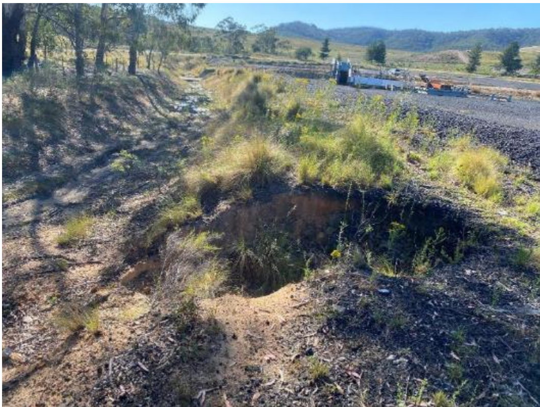
Photo 16 - Area of Erosion at the Main Drain at Kerosene Vale
