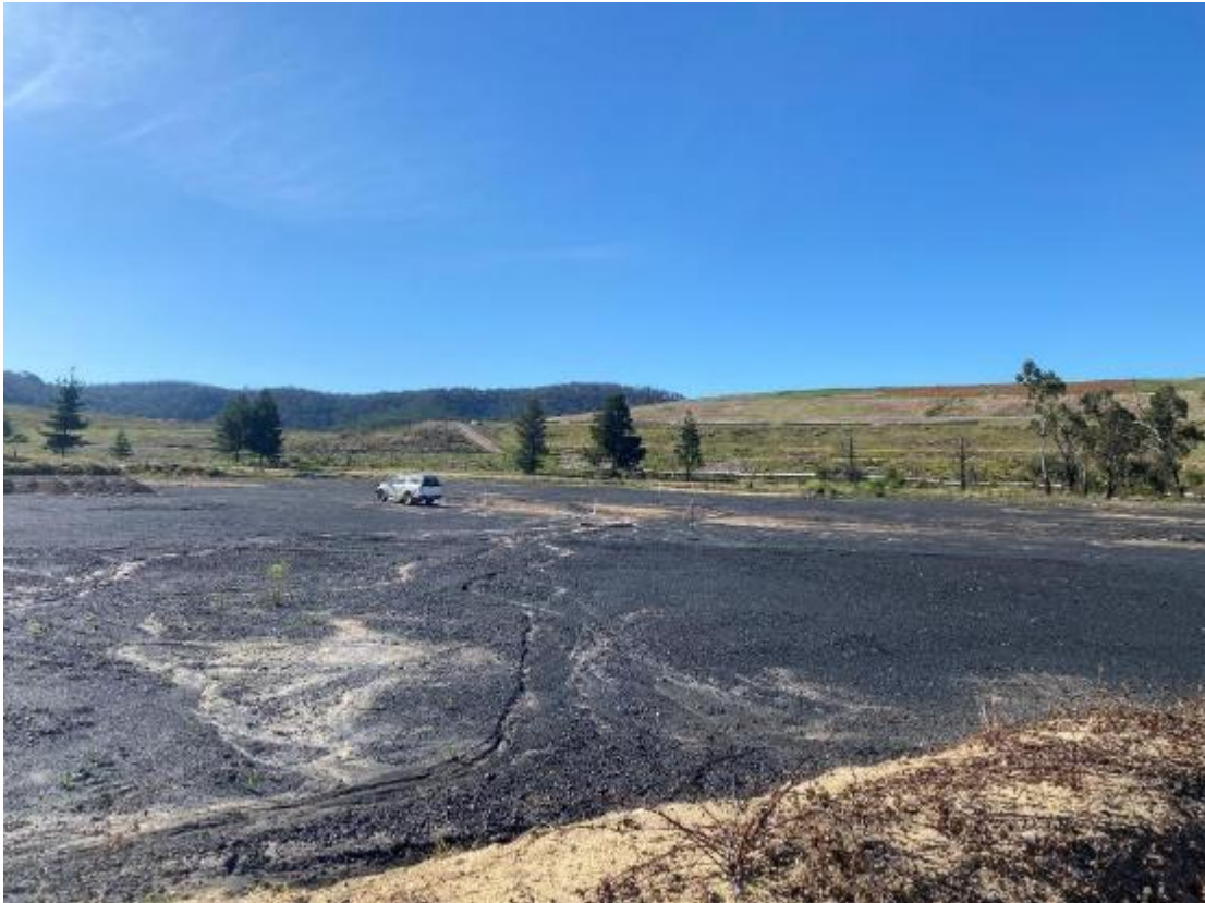
Photo 08 - Water Management Works are Required to not Accept Water from GPM Land at Kerosene Vale
