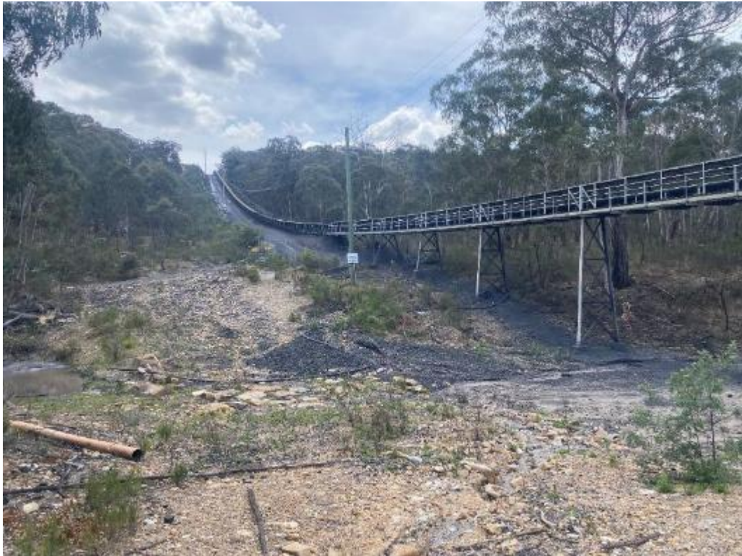
Photo 11 - Further Work Is Required on the Drain on the Left-Hand Side of This Photo
