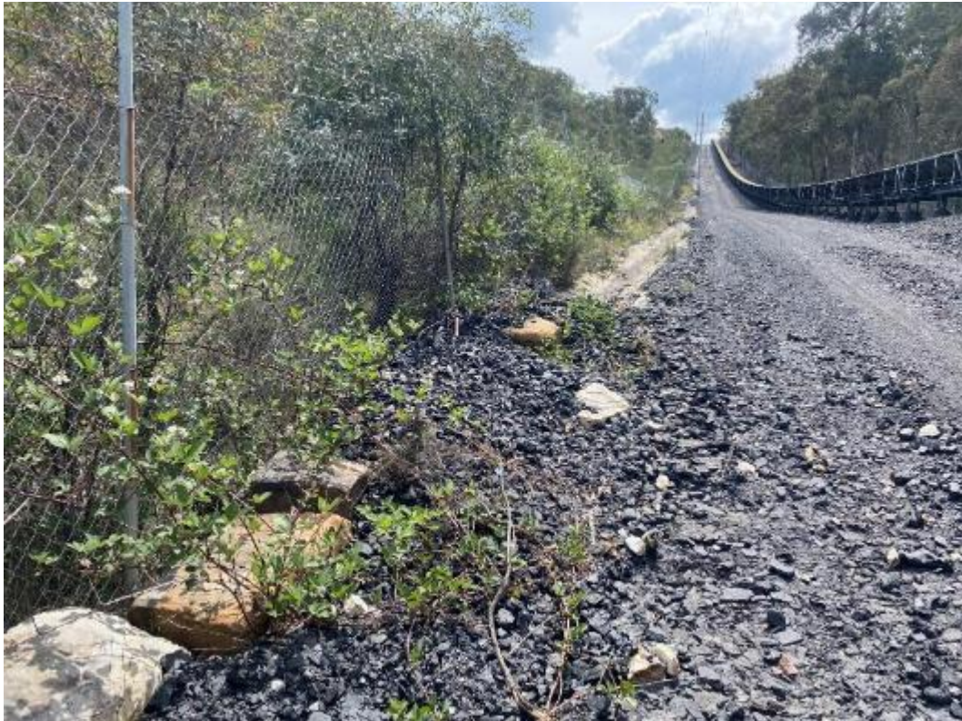
Photo 15 - Further Works Required in Drain to ensure it flows directly to the dirty water management system
