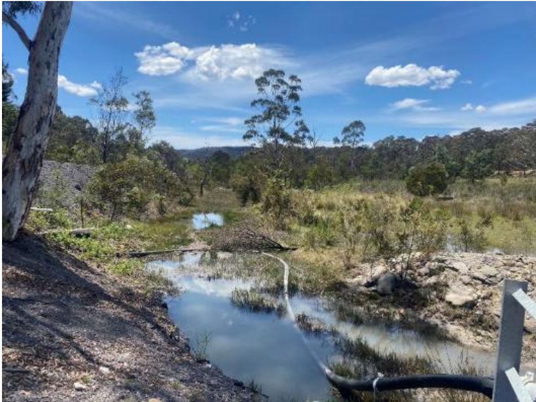
Photo 05 - Stable Cleanwater Drain at Site
