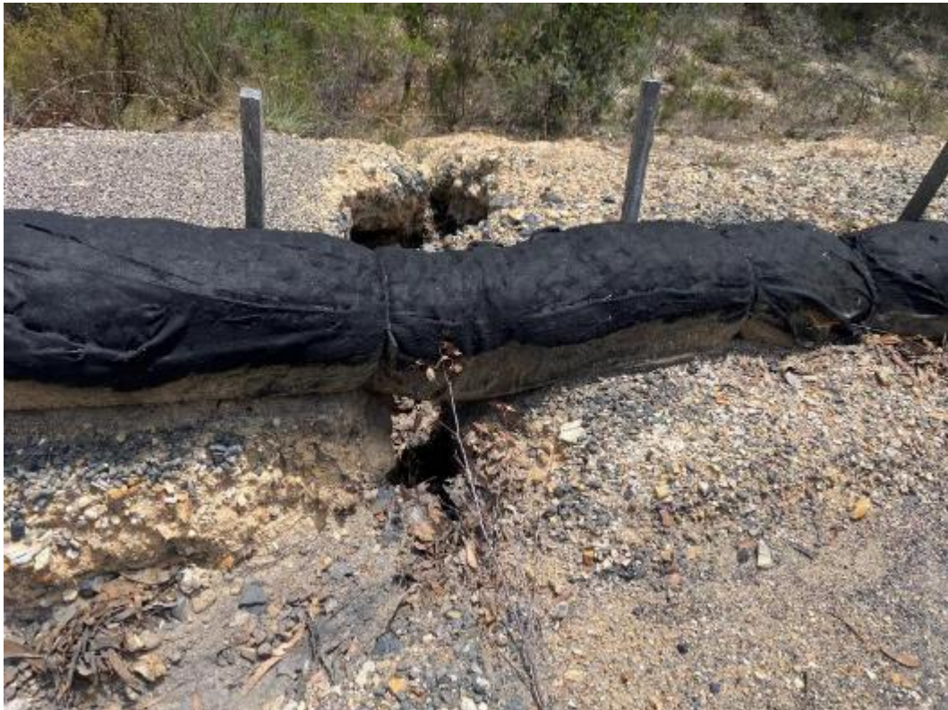
Photo 12 - Minor Erosion Where Carbonaceous Material Can Leave Site Near Transfer Area
