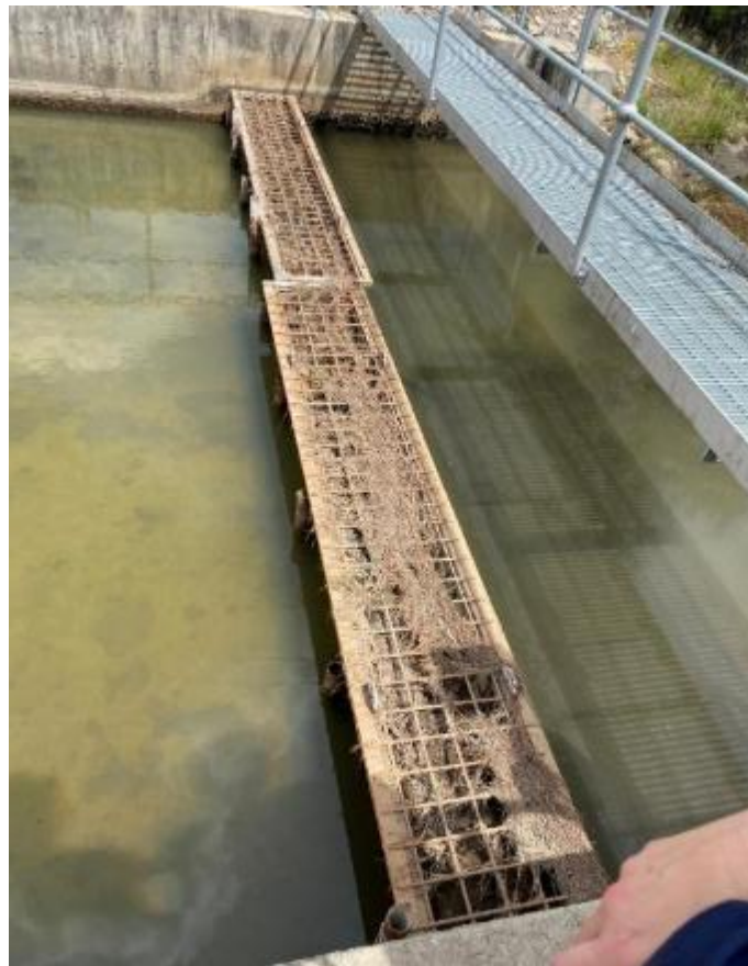
Photo 02 - Hay Bales Trap Needs to be Replaced at LDP
