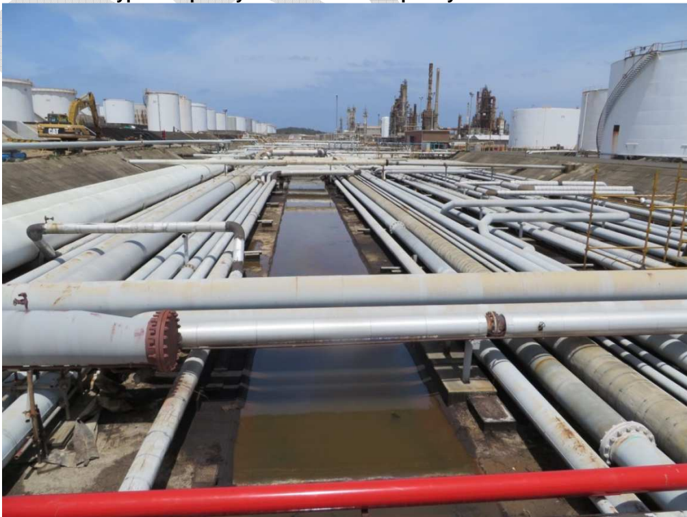
Figure 5-2 Photo of Typical Pipeway Section – Main Pipeway
