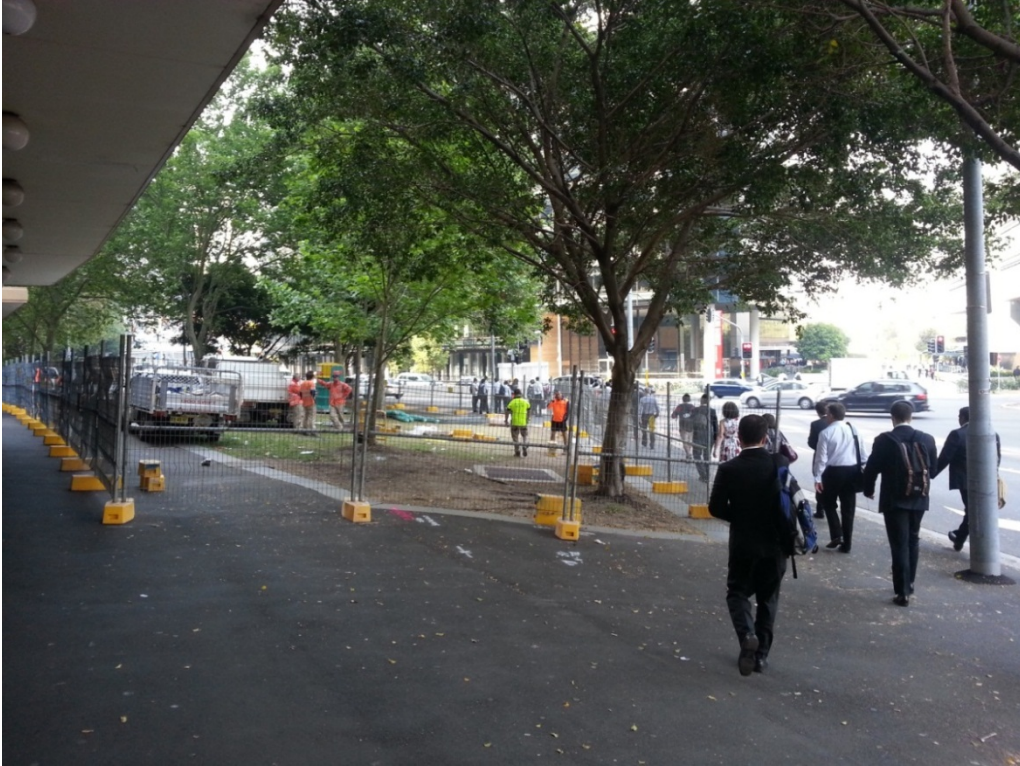
Figure 7. Remedial works to rectify pedestrian inadequacies Source: City of Sydney
