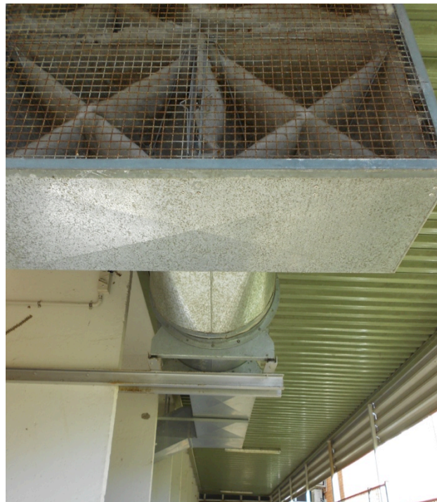
Figure 2 – Existing noisy fan at north of existing ward building
