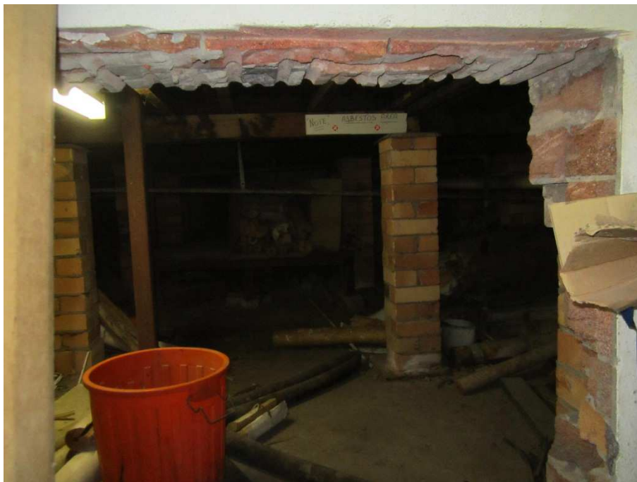
Photograph 4, Photograph shows the surface soils beneath the raised timber flooring that present in the northern part of the laundry building.
