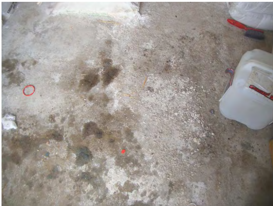
Photograph 8, Photograph shows some minor surface staining on the concrete flooring in the former fumigation building.
