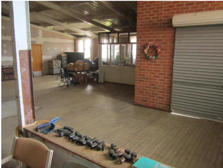
Photograph 3, Photograph shows the raised timber flooring in the north part of the former laundry building.
