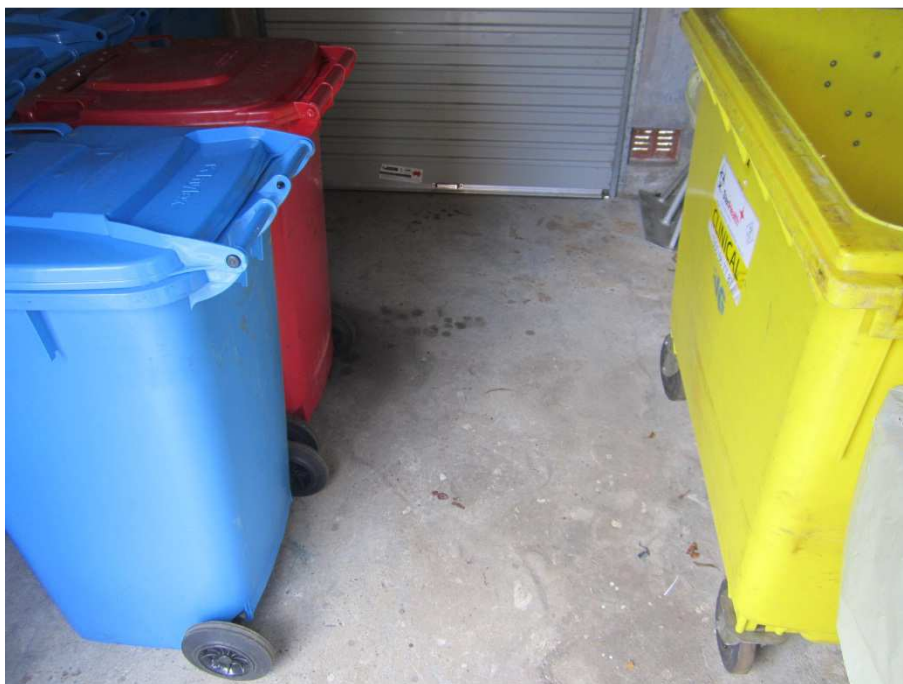
Photograph 6, Photograph shows concrete flooring in former Coke storage building in relatively good condition with minor staining present.
