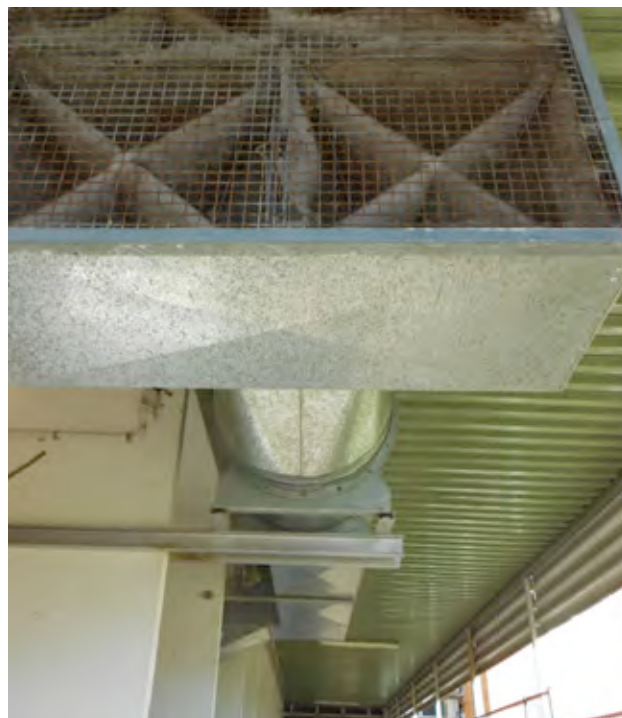
Figure 3 – Existing noisy fan at north of existing ward building
