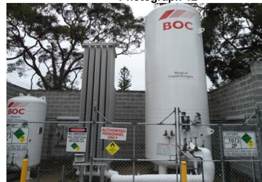
Oxidising Gas Tanks Storage
