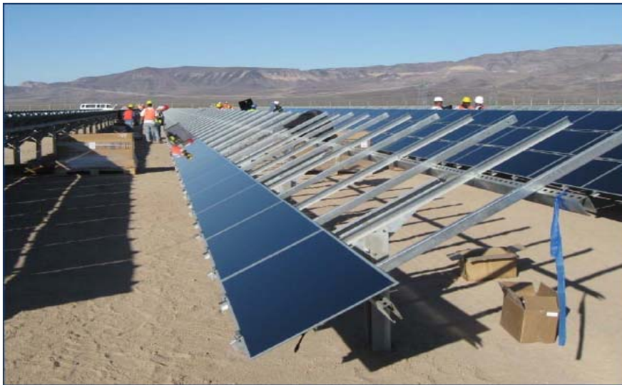
Figure 3-3 First Solar modules and racking tables.
