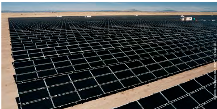
Figure 3.1 Typical solar arrays (image courtesy First Solar)
