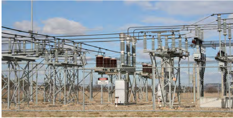
Figure 3.2 Typical substation found in Australia
