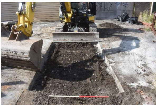
Figure 2.12 Trench 02 mid-excavation, showing spatially constrained nature of 1–3 Bank Street Courtyard. 1m scale.
