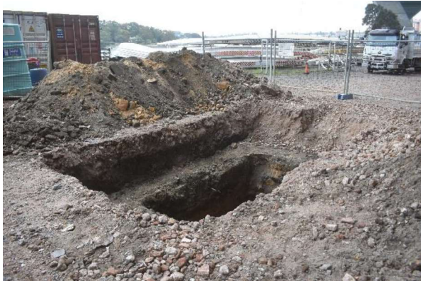
Figure 2.20 Trench 4, facing west, showing stepped nature of the trench due to deep excavation.
