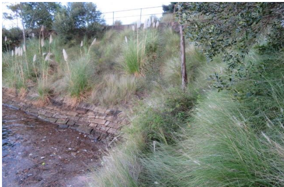
Figure 2.15 Junction between the sandstone-faced eastern abutment of Glebe Island Bridge and 1A Bank Street.
