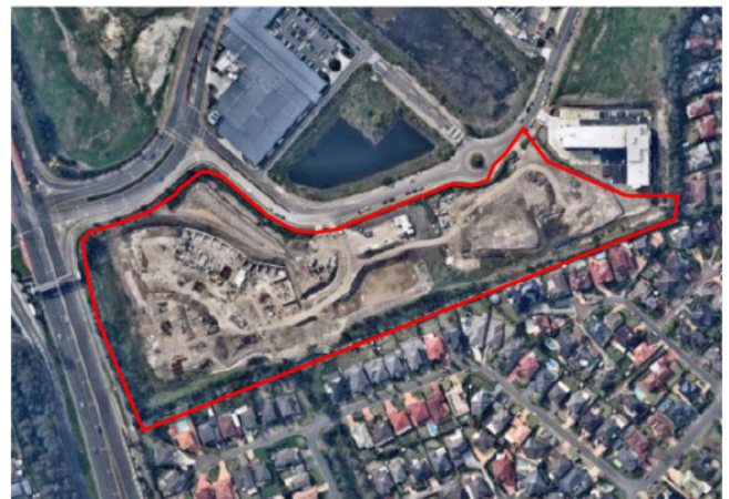
Figure 20 – 2016 aerial showing development occurring the subject area and construction of deep drainage basins.
