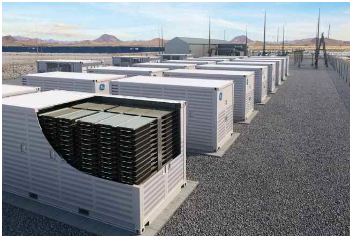
Figure A.10 Typical Battery Storage Arrangement
