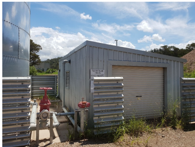
Figure 4 – Pump Room Enclosure
