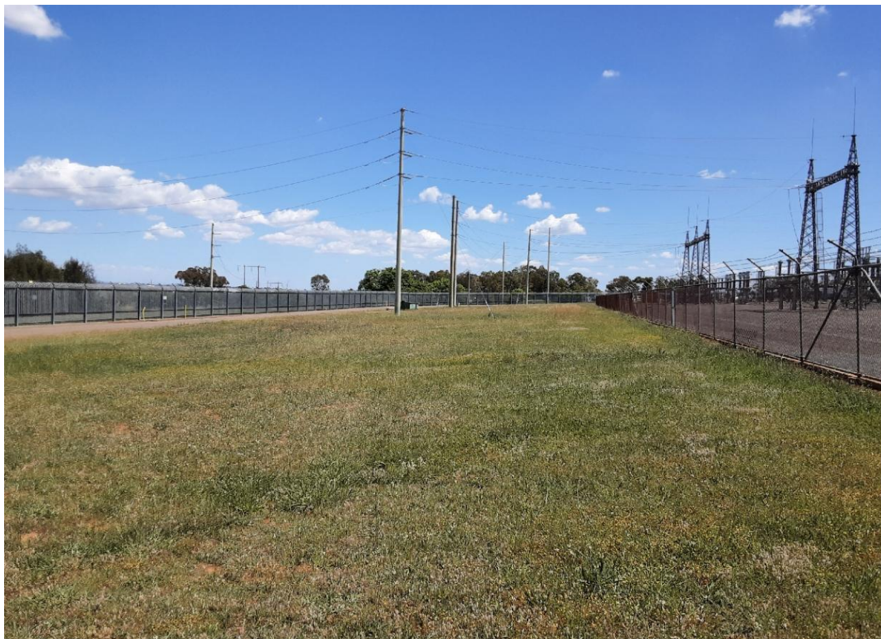
Photo 1 PCT 599_DNG_Low within the TransGrid substation
