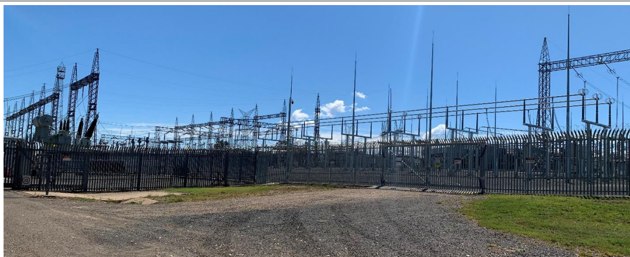
Figure 10: Existing Tamworth Substation Compound (Source: Equis, 2024)
