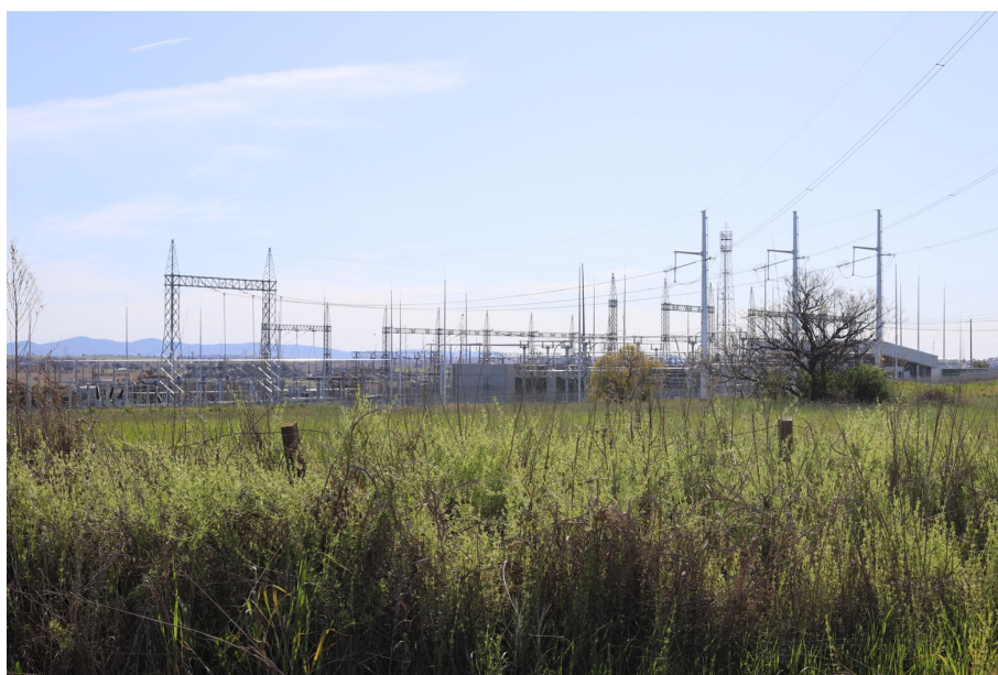
Figure 3-9: Existing TransGrid Tamworth Substation
